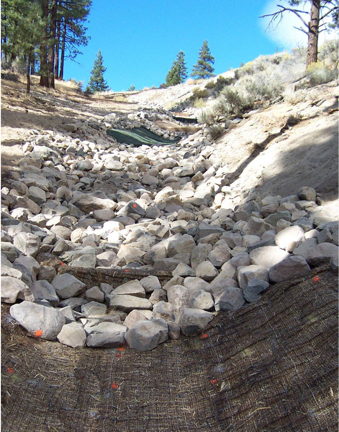
Figure 4.19 Completed installation of rip rap and North American Green SC250 in lower field plot (October 2003).
