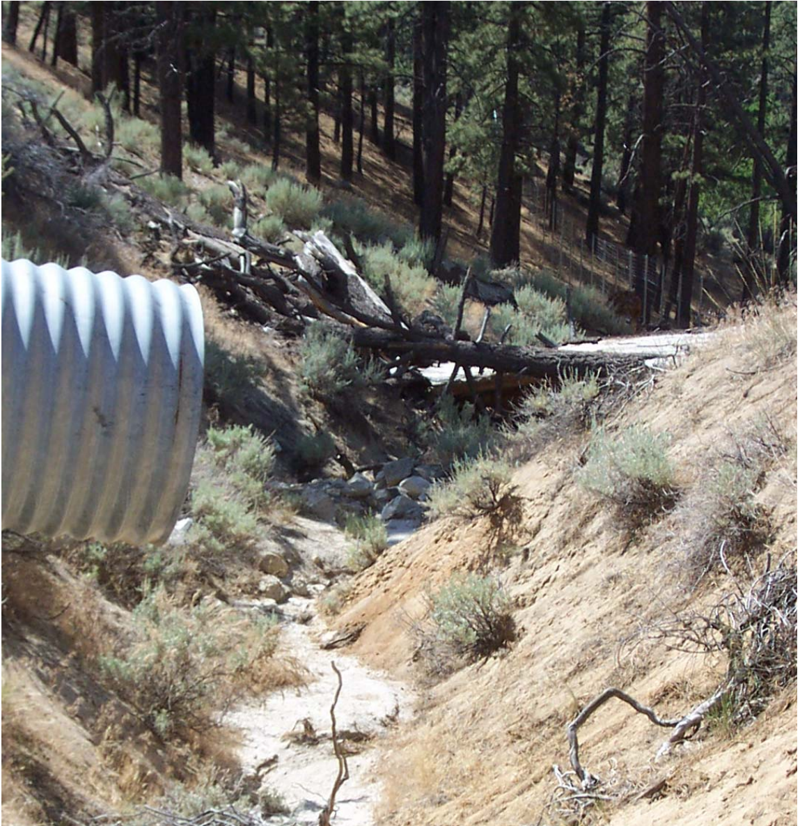
Figure 4.11 Original conditions at culvert outlet before channel reconstruction and installation of field plots.
