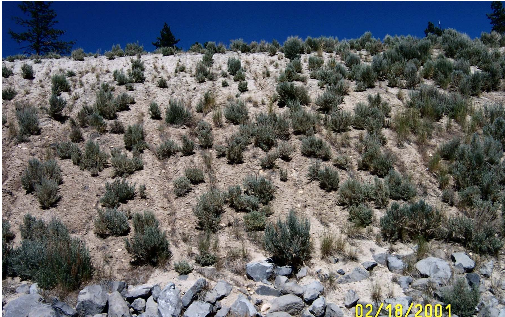
Figure 2.8 Rill erosion, U.S. Highway 50 roadway embankment, Clear Creek watershed.
