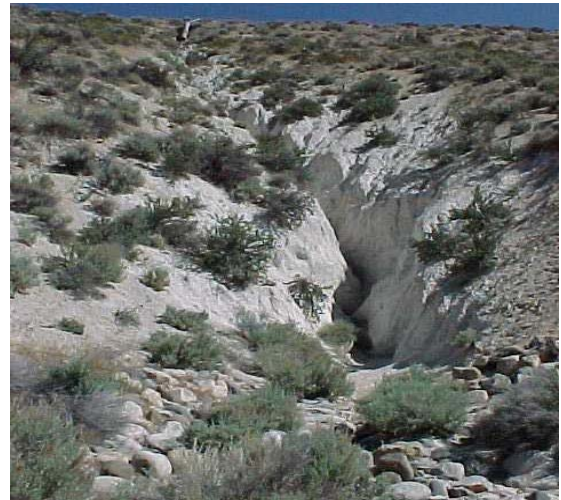
Figure 2.24 Gully erosion from culvert.
