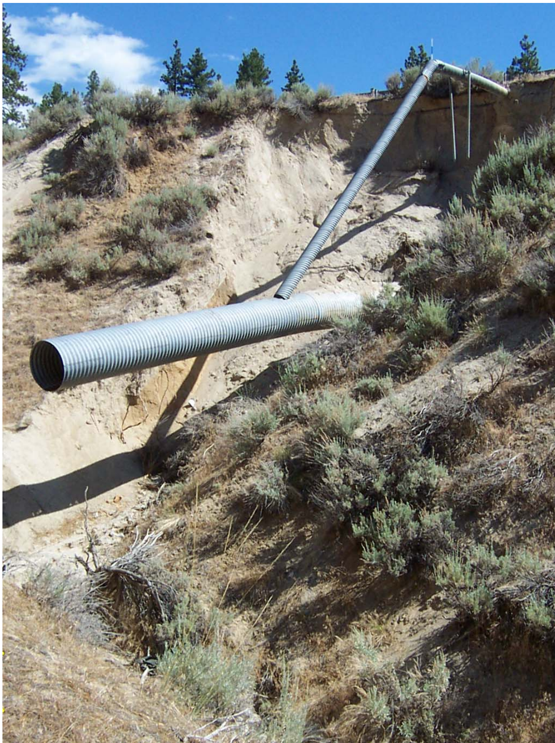
Figure 4.10 Uncontrolled erosion at culvert outlet before channel reconstruction and installation of field plots.
