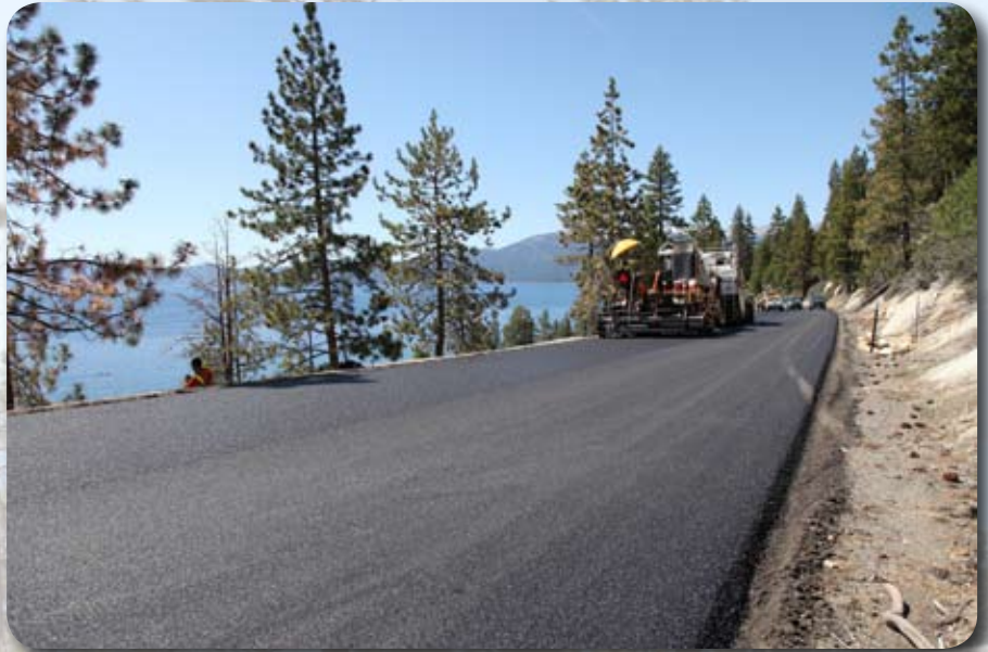
Scenic Lake Tahoe is the perfect backdrop for a near-completed State Route 28 project as pictured in late May.
