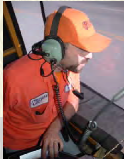
NDOT maintenance professionals use a dedicated eye while operating machinery to restripe Nevada freeways for better visibility and safer travel.
