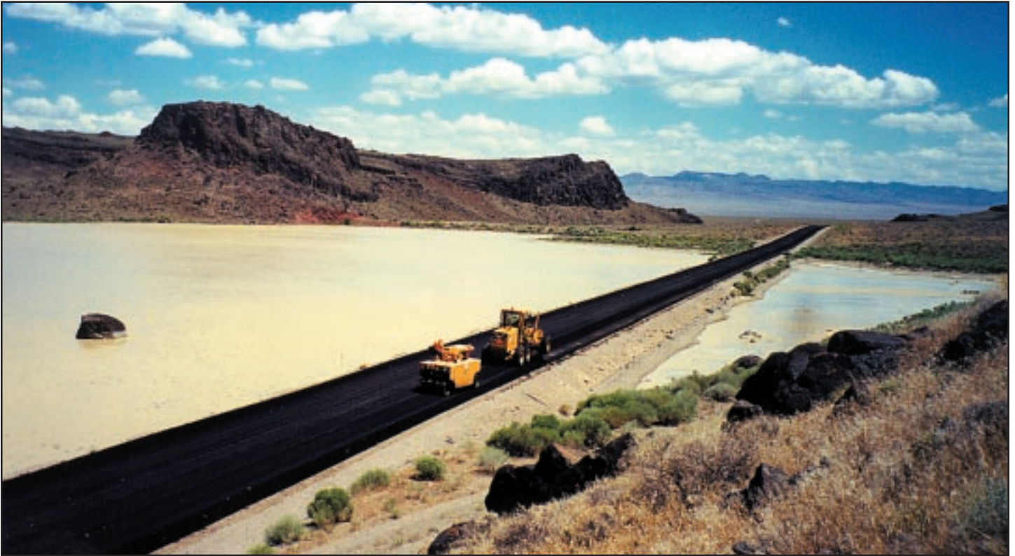
After a desert rain, crews pave the Blue Jay stretch of the E.T. Highway. Below: The natural surroundings of Blue Jay include the NDOT oasis, deer that frequent a nearby spring, mineral waters at Warm Springs and a Russian Juniper they said could not survive the terrain.
