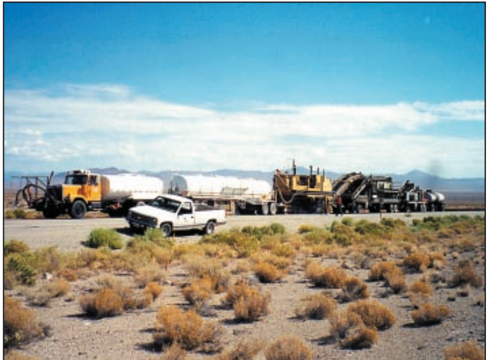
The cold recycling train's milling machine, crusher and pug mill in action.
