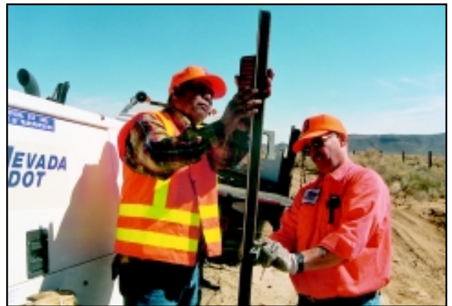
INSTALLATION —The Strieter reflectors are mounted on posts away from the shoulder of the road, so the posts themselves are not a hazard to motorists or maintenance. Doing the installation work are highway maintainers Byron Fillmore and Joe Smaltz from crew 272.
