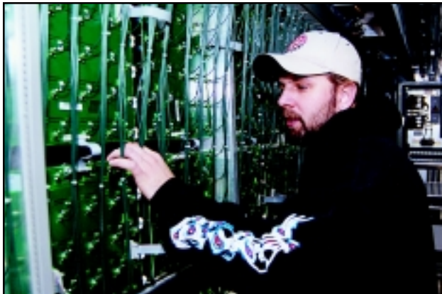
SMOOTH INSTALLATION—New changeable message signs are going into service in Las Vegas and Reno. The signs will alert motorists to delays, weather conditions and chain or snow tire requirements. Jody A. Lett of the sign's manufacturer, Dambach, Inc., puts one of the big signs through its paces.
