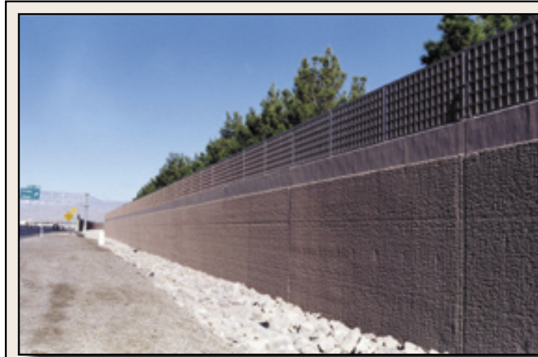
LIGHT FRIENDLY- The sound wall near Craig Road on US-95 is topped by a section of polycarbonate plastic that lets light through, but diminishes sound.
