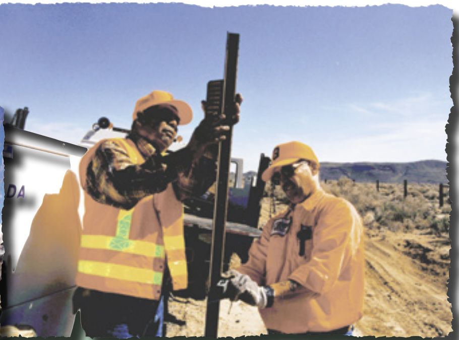
INSTALLERS—Strieter reflectors are mounted on posts away from the shoulder of the road so the posts themselves are not a hazard to motorists or maintenance work. Doing the installation are highway maintainers Byron Fillmore and Joe Smaltz from Crew 272.
