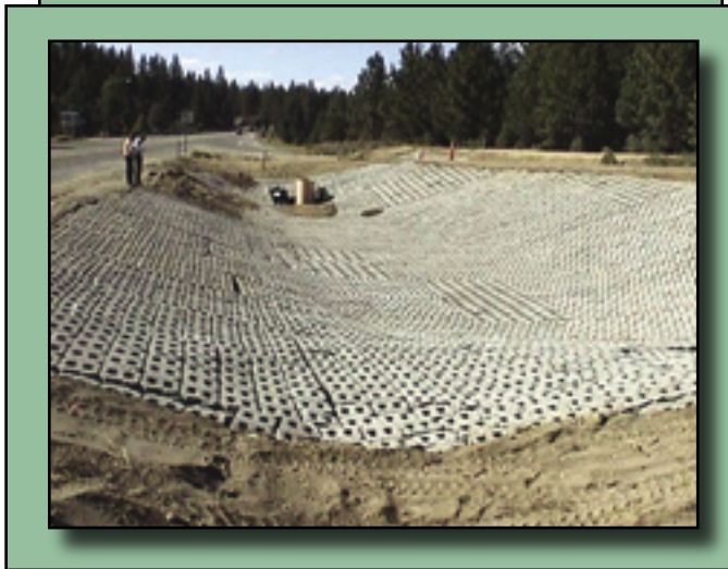
A sediment basin in the Lake Tahoe area—Articulated concrete blocks are used as flexible lining for erosion control where deep or rapid water may cause a stability problem.
