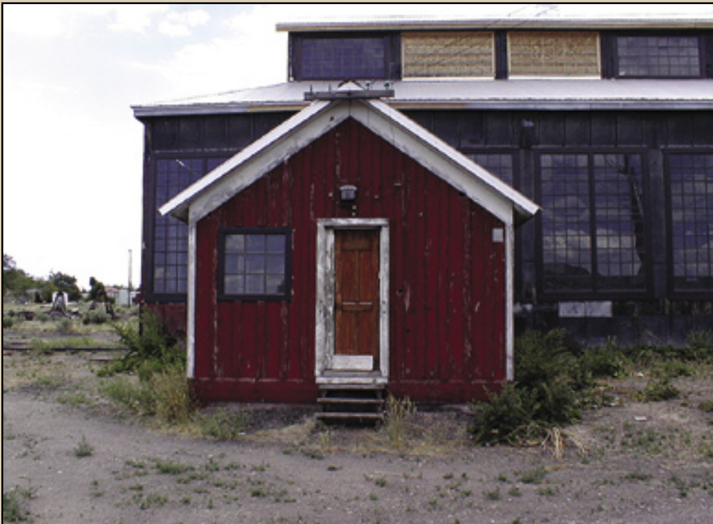
RESTORATION—The White Pine Historic Railroad Foundation has done an excellent job bringing back the rail line established by Kennecott Copper. The coach shed was in danger of collapsing prior to the restoration work.
