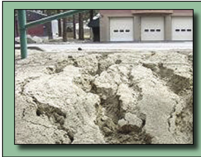
An example of major rilling caused by impervious surface contact with unprotected soil. After repairing the slope, the area might be covered with an erosion control blanket and seeded.
