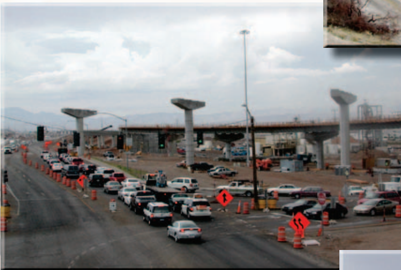
WORK IN PROGRESS—Piers for the flyover at the I-215/515 Interchange show the promise of leaving signal lights and cross-traffic behind. Reconstructing the interchange and extending the Southern Beltway is an $82 million project pending. Actual freeway widening is on hold.
