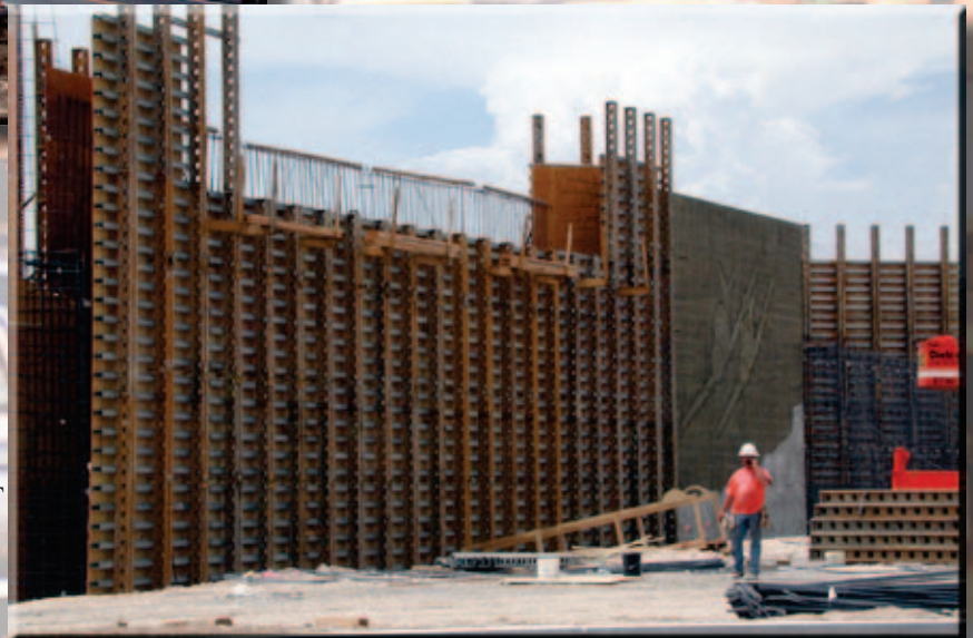
FULL INTERCHANGE—I-15 at Lamb Boulevard will be upgraded to a full interchange at a cost of $17.5 million. The contract was awarded in November and is scheduled for 300 working days.
