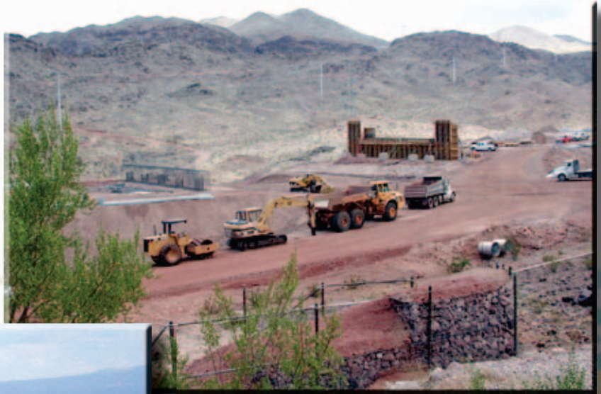
HOOVER APPROACH—The Nevada and Arizona bridge approaches are under construction, with the Nevada approach costing $32 million and the Arizona construction to cost $22 million.
