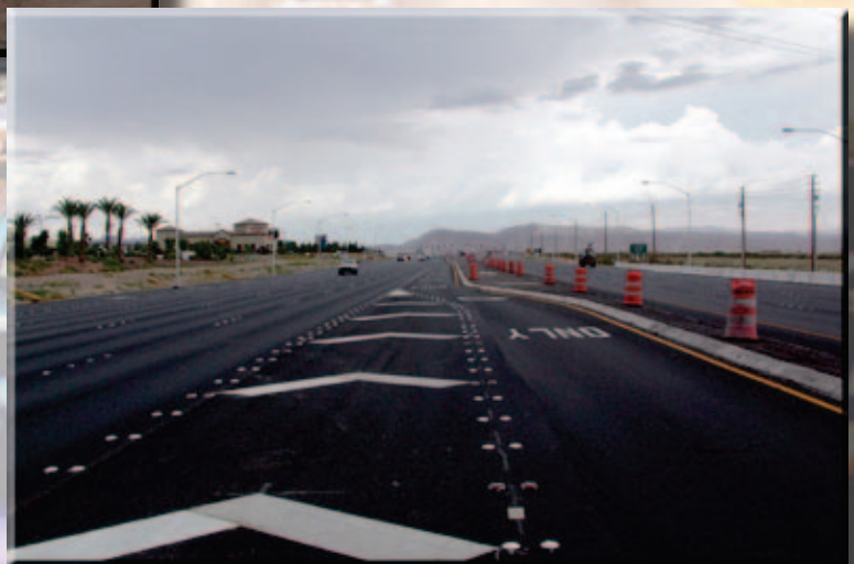
SMOOTH SAILING—Widening of the St. Rose Parkway is nearing completion. In addition to increasing the number of lanes to as many as eight, the interchange with I-215 is being reconstructed, including signals, lighting drainage and bridges. Cost of the project is $20.1 million.
