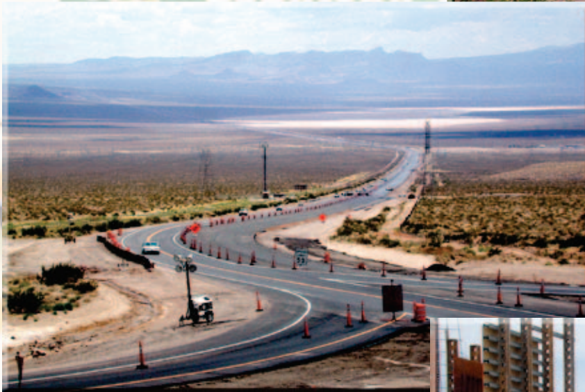
CORRIDOR IMPROVEMENT—Widening of US-95 from 18 miles north of Searchlight to Railroad Pass is nearing completion. The $23.7 million project was preceded by widening of a stretch of highway from Searchlight to the new project in 2003.
