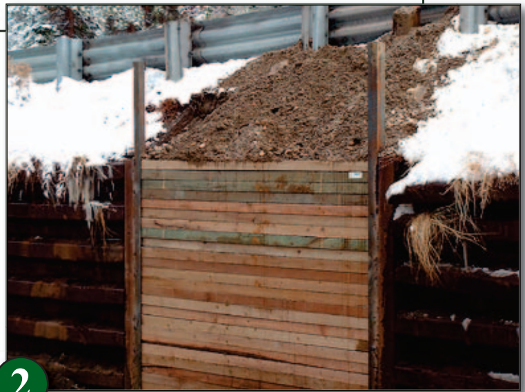
TEMPORARY FIX—Wood is used to patch up the bin wall.
