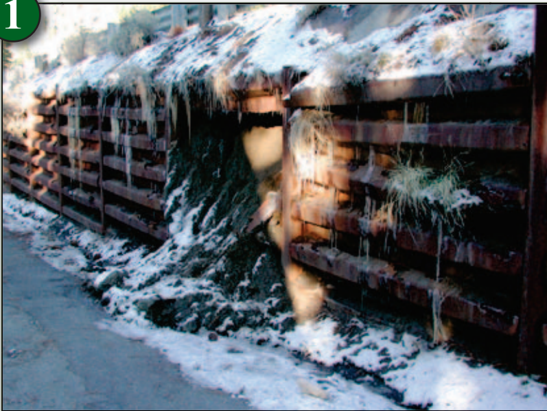
BEFORE—A deteriorating bin wall for a third of a mile along US-50 near Cave Rock required a $2.7 million replacement and drainage improvements.
