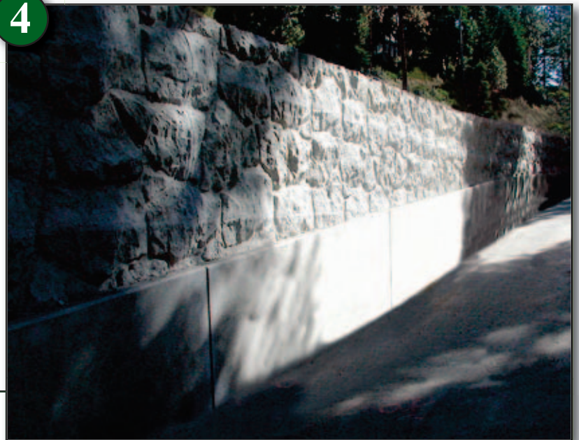
AFTER—Appearance of stone work adds to the aesthetic appeal of bin walls.
