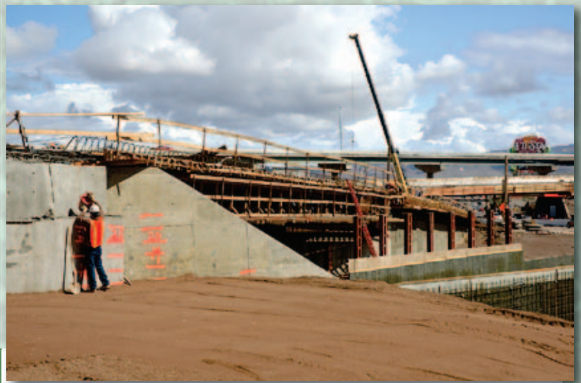
MAKING PROGRESS—The falsework on the ramp from north I-515 to West I-215 indicates the progress being made. At far right is more falsework that is part of bridge widening over I-515.
