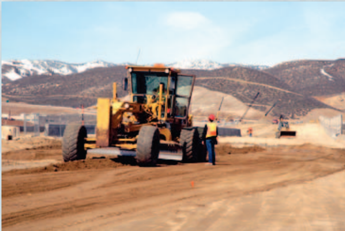
BLADE IT FLAT—Fine grading is done on the embankment south of the Arrowhead Drive Bridge structure, part of the Carson City Freeway project.
