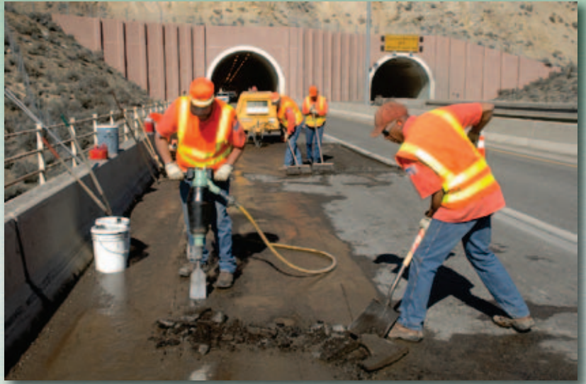
A LITTLE OFF THE TOP—Cracked asphalt is cut, jack hammered, dug up and removed from a bridge deck outside the Carlin Tunnels. Crews 350 and 355 from Elko do the work.
