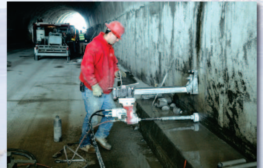
DRILLING —A worker with Diversified Concrete Cutting drills a weep hole for draining the tunnel.
