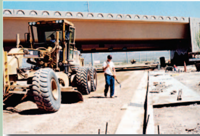
FINE GRADING—Sidewalks are being poured, trees are being planted and scrapers are making their final passes prior to paving at the Lamb Boulevard Interchange. The structure should be completed by August.
