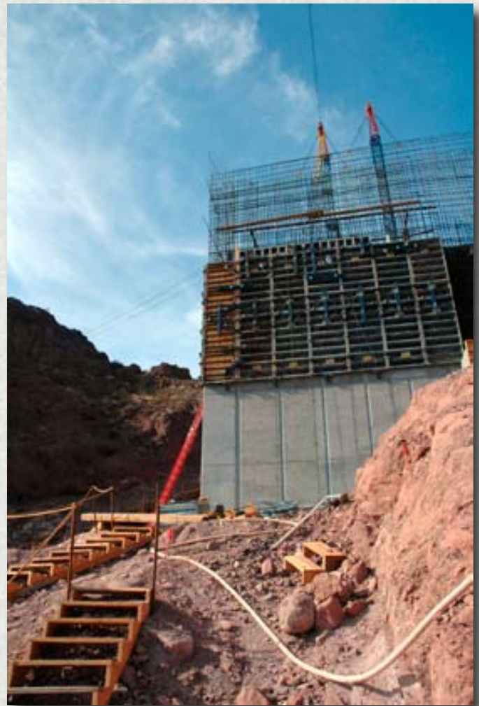
FOUNDATION WORK—With the approaches completed from Nevada and Arizona, the next step is to build the bridge structure over the Colorado River.
