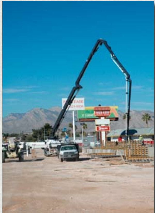
US-95—Years of work to widen US-95 through Las Vegas are coming to fruition, including this area at Jones and US-95 where a snorkel truck is being used to pump in cement to provide drainage structures.
