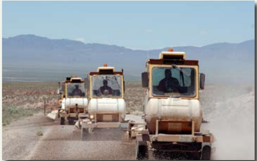
CHIP SEAL—NDOT workers sweep up loose chips after a chip sealing project in rural Nevada. By using asphalt overlays, slurry seals and chip seals, the department is able to delay expensive reconstruction.
