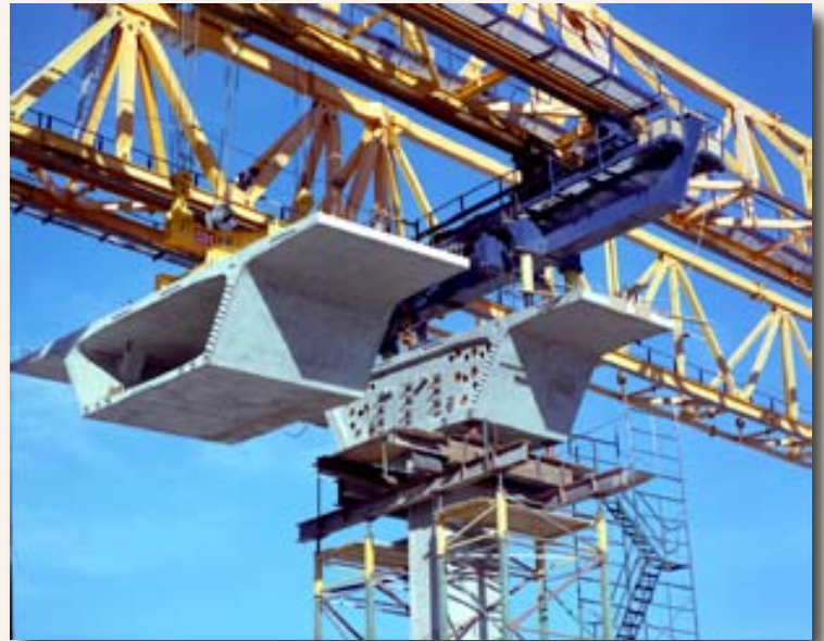
MASSIVE CONSTRUCTION —At 66 tons per segment, and 675 pre-cast bridge sections, the construction of the Las Vegas Spaghetti Bowl in 1999 was a huge project with eight freeway to freeway flyovers. It was the first Nevada project to use large pre-cast bridge segments.
