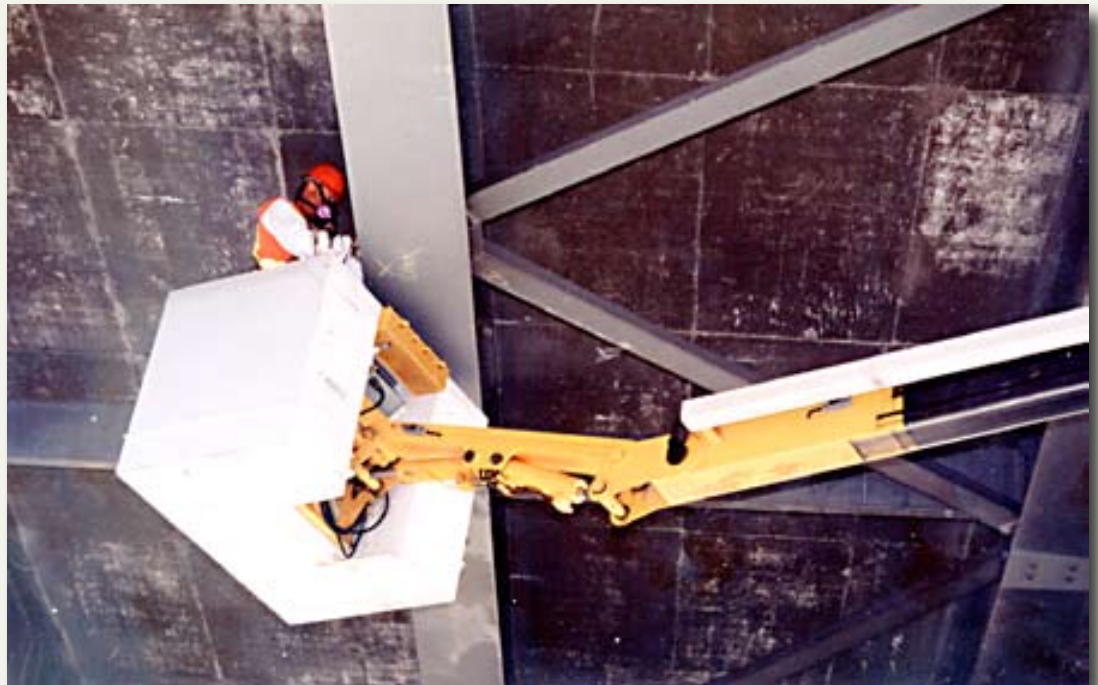
BRIDGE INSPECTION--All of the state’s public bridges, not just those owned by NDOT, undergo an inspection every two years. Every four years each bridge received an in-depth inspection where hundreds of measurements are taken. Larger structures, like the one shown, are inspected from a boom truck.
