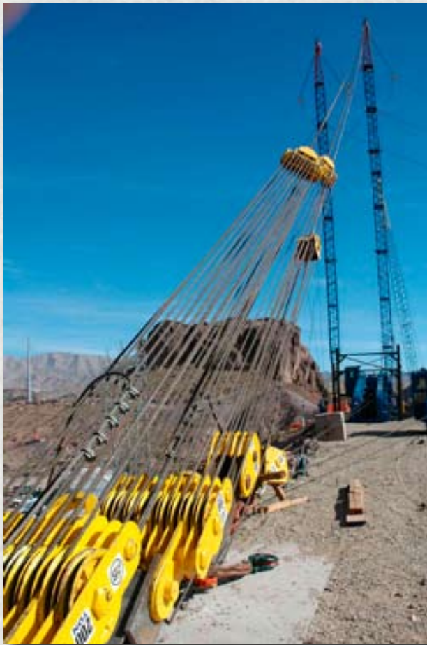
COLORADO BRIDGE—Cables and pulleys support the first temporary towers in the construction of the bridge bypassing Hoover Dam. Completion is scheduled for 2008.
