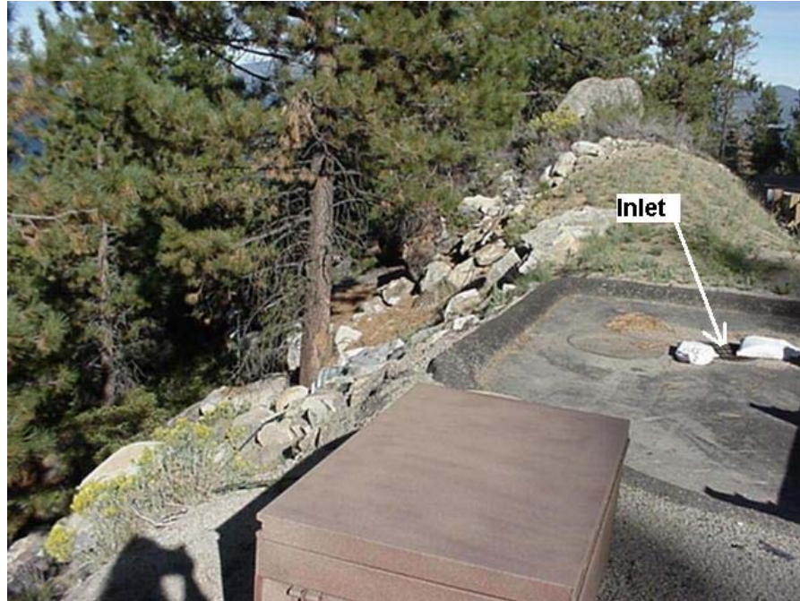
Figure 7.2. NDOT 4 Study Site, Stormceptor® unit.
