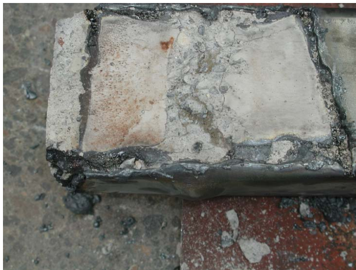
Figure 3-20: Concrete Exposed at Location of Buckling
