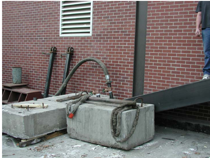
Figure 2-16: Pump attached at the bottom of the tube and pumping the grout mix up
