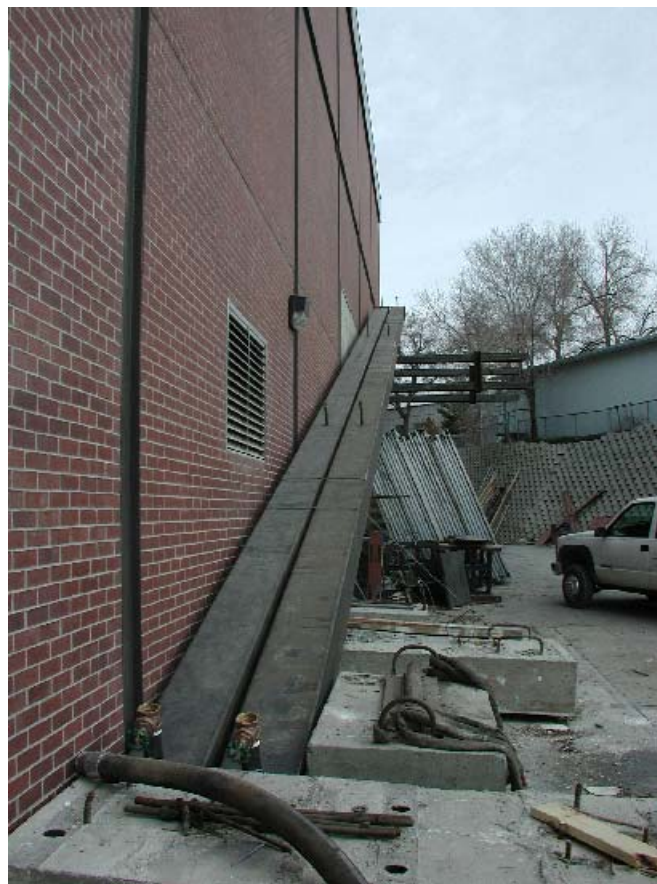
Figure 2-17: The 80-ft Structural Steel Tubes Prior to Being Pumped Full with the Grout Mixes
