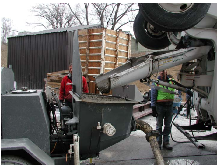
Figure 2-11: Trailer Line Pump
