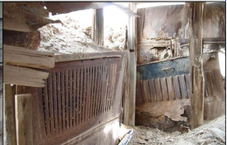
Reprioritized louvered automobile hoods used to short up walls in of the features at the Double O Mine site. Photo by Sean McMurry.
