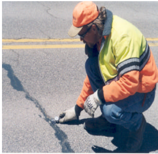
Figure 2. Measuring crack size with a micrometer with precision of 0.001 inches.
