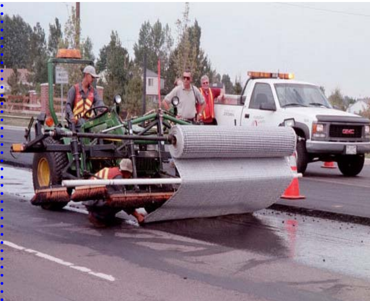
Paving grid T1343 installation in Denver, Colorado. For the NDOT project, the grid will be supplied without the light weight polyester fabric.
