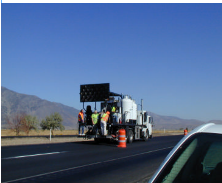
Photo 2. Installation of LPM 1200 polyurea marking using mobile, truck mounted and self-contained pavement marking machine.
