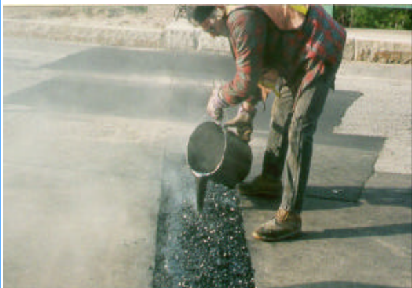
Photo 4. Field installation of the A.P.J. system from SSI on a Texas bridge.
