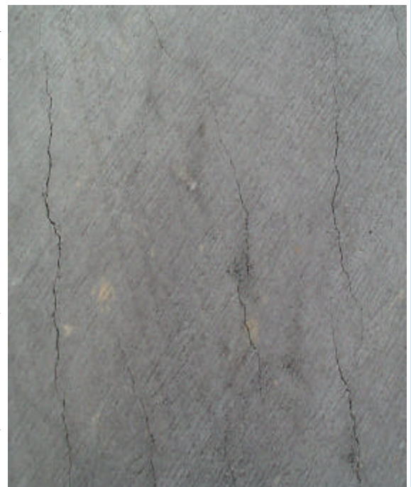
Photo 1. Extensive cracks in the mid-section of the deck.
