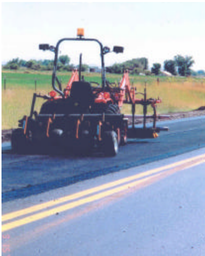
Photo 6. Installation of the GeoGrid fabric to reinforce asphalt concrete overlays in pavement construction.
