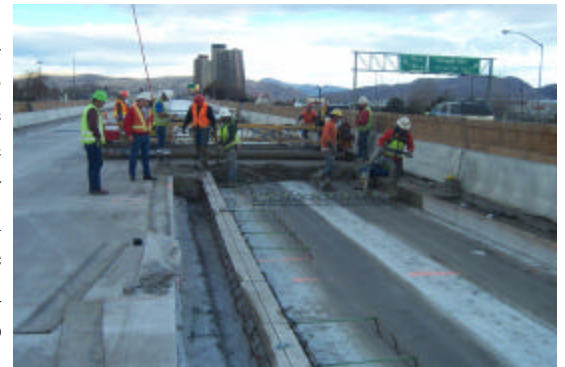
Photo 4. The Construction Crew "Pouring" the Trench Drain and New Lane on I-80 Project.
