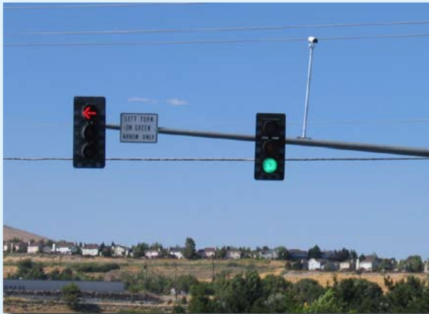
Figure 1: Shows the typical permissive left turn display with a red arrow. The green ball means that the driver turning left must yield to on-coming traffic.
