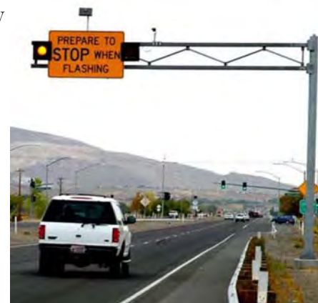
Figure 11. Flashing warning lights at Johnson Lane.
