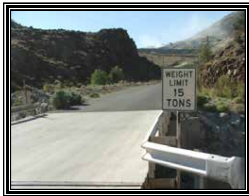
Example of Structurally Deficient Bridge
