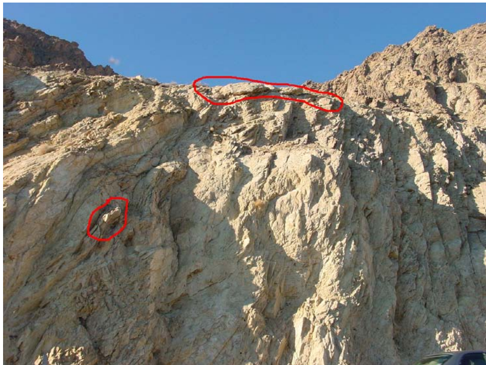
Fig 22. Milepost 63.89 showing fractured bedrock wedge and soil overhang. Note highly fractured bedrock across cut face.
