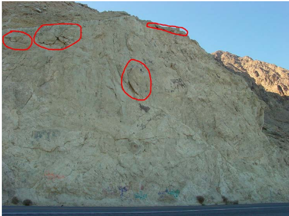
Fig 2. Milepost 62.9 showing fractured rock and overhanging material.
