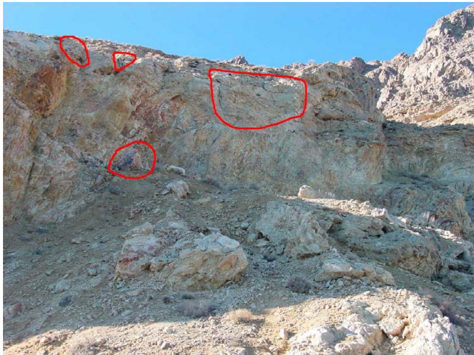
Fig 12. Milepost 63.55 showing fractured cemented soil on top of cut and large rock perched on slope.
