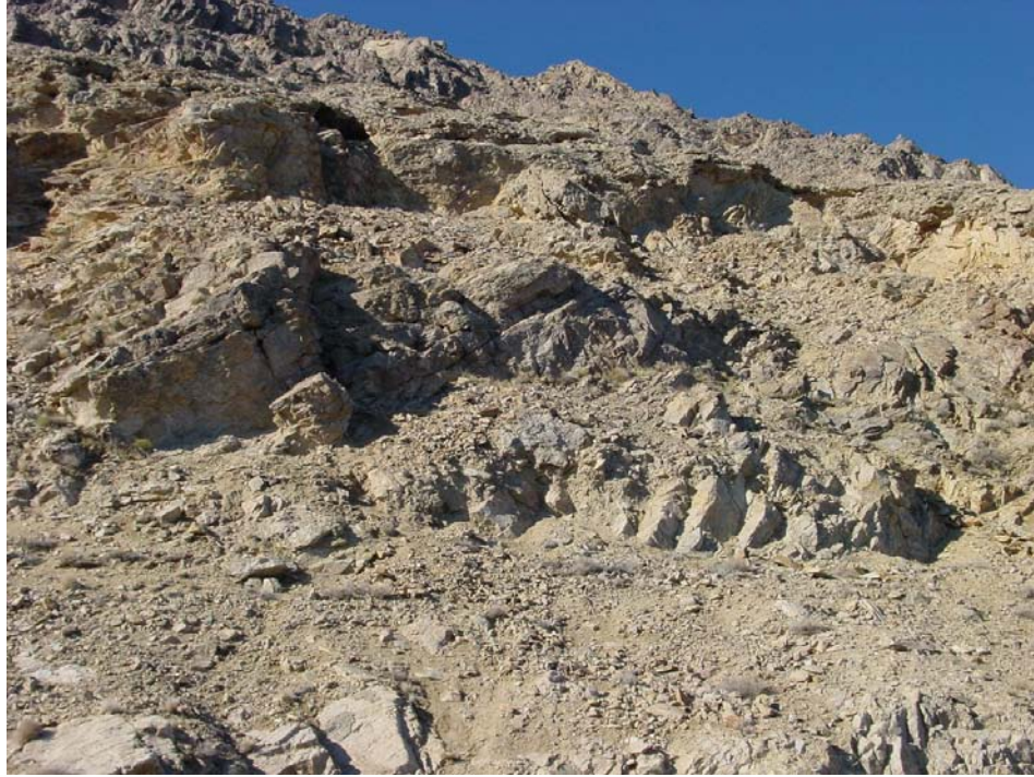
Fig 13. Milepost 63.61 showing large volume of unstable rocks perched on slope.
