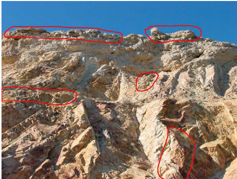
Fig 14. Milepost 63.67 showing fractured rock wedge, over steepened degraded bedrock and cemented soil overhangs.
