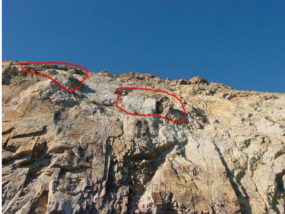
Fig 7. Milepost 63.36 showing failed rock mass perched on rock face and overhang at top of cut slope.
