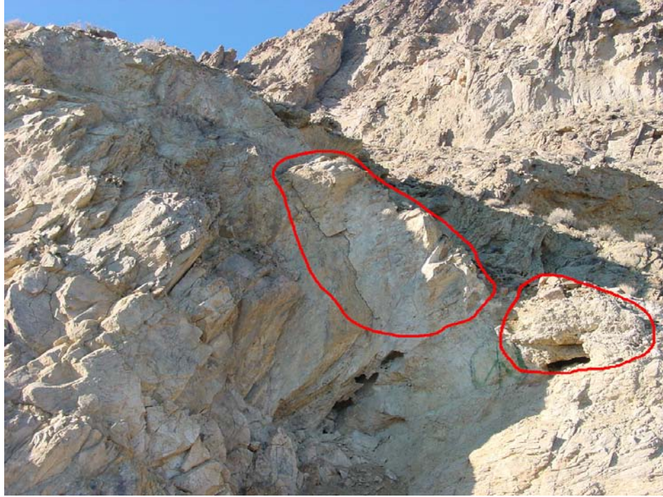
Fig 25. Milepost 63.96 showing large bedrock wedge and soil overhang.
