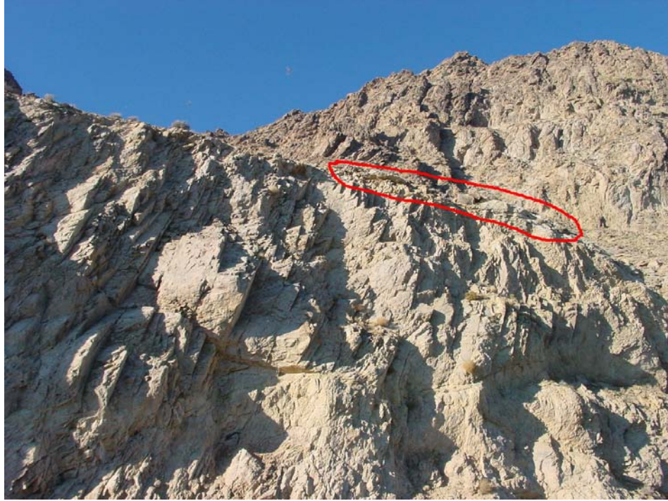
Fig 23. Milepost 63.91 showing loose rocks perched at top of slope. Note highly fractured bedrock with many open fractures across cut face.
