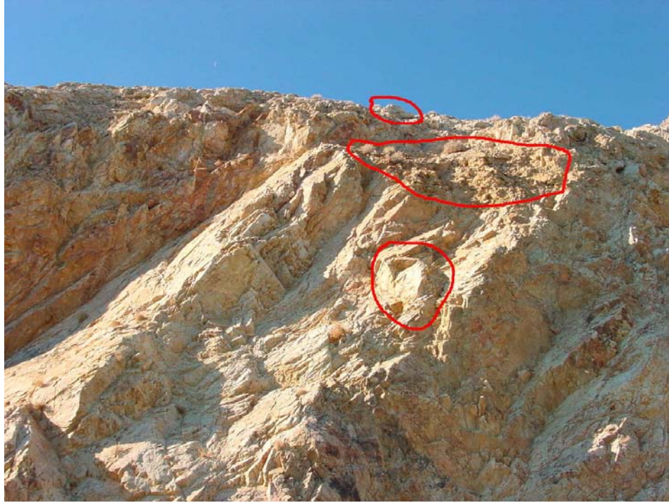
Fig 11. Milepost 63.53 showing large rock wedge, loose rocks perched on slope face and large rock at top of slope.
