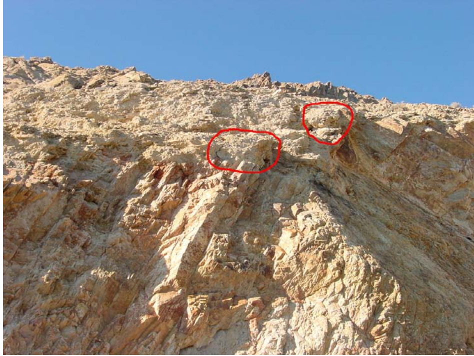
Fig 17. Milepost 63.74 showing fractured soil overhangs. Note intense fracturing of bedrock across cut face.
