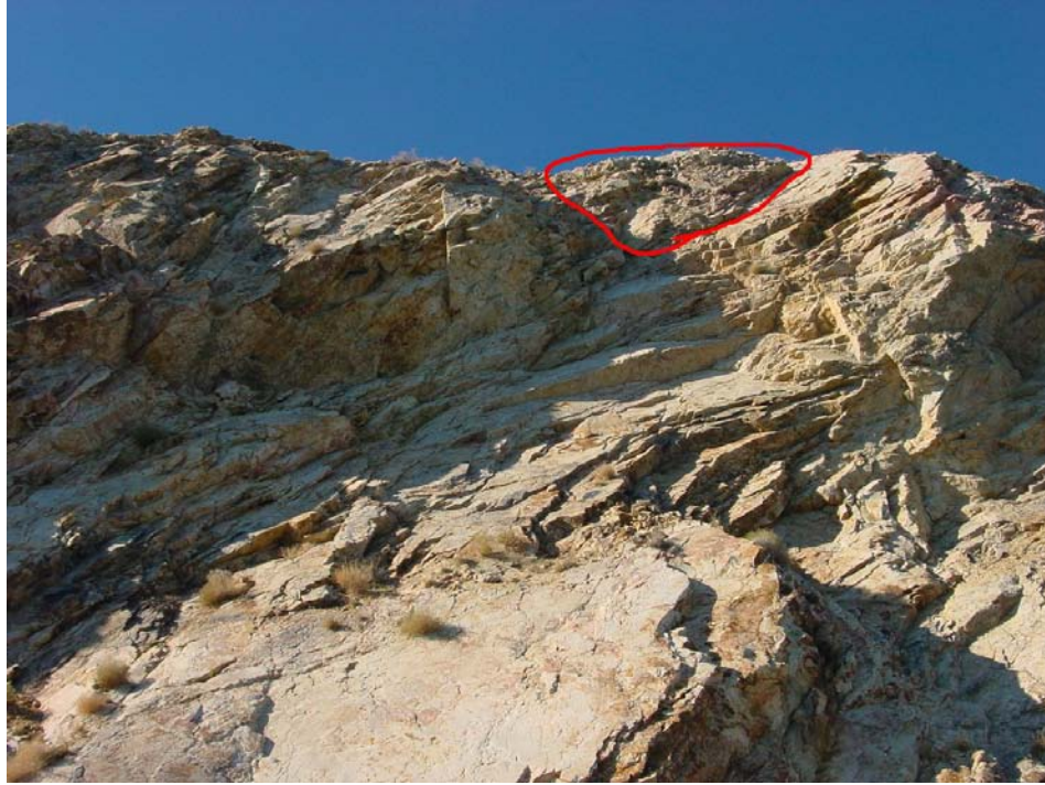
Fig 9. Milepost 63.48 showing poorly cemented soil mass at top of slope. Note many rock fractures across cut face.
