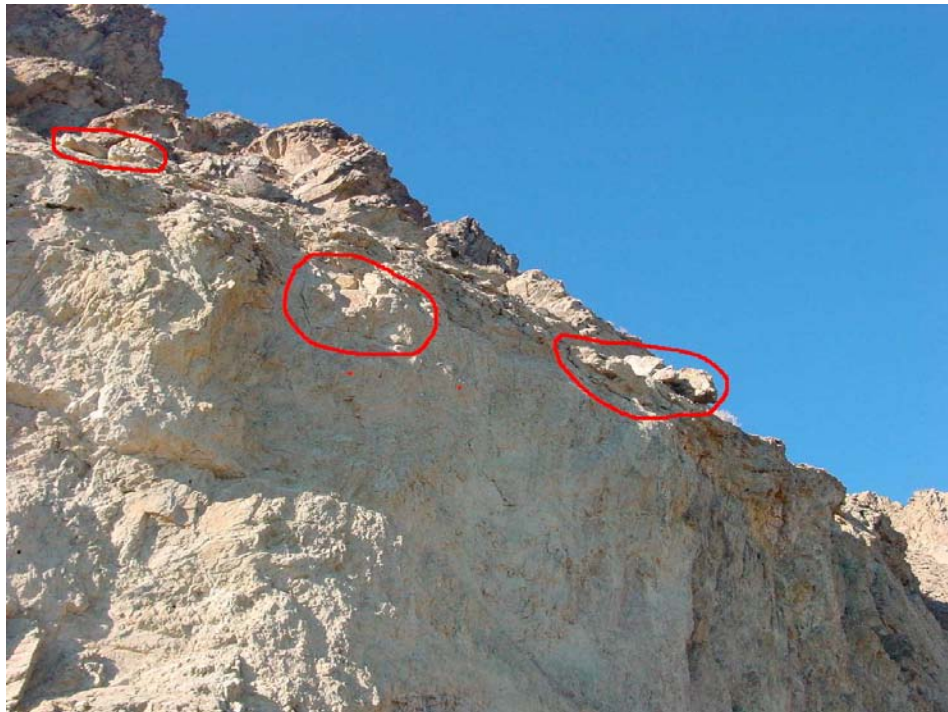
Fig 26. Milepost 64.07 showing fractured rock and large loose rocks on top of cut slope.
