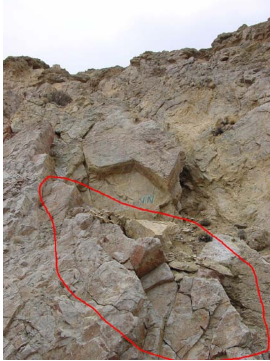
Fig 1. Milepost 62.8 showing loose rocks and fractured rock to be scaled.
