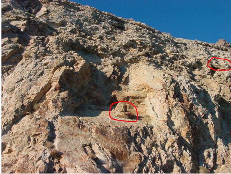
Fig 19. Milepost 63.76 showing perched loose rock and unstable wedge of cemented soil.
