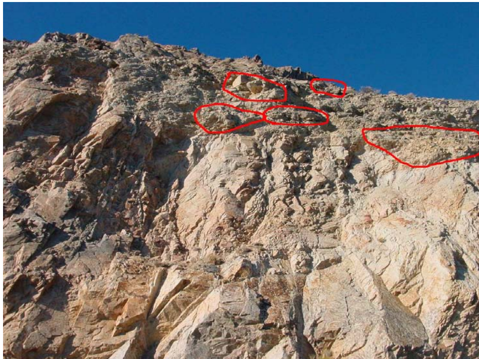
Fig 16. Milepost 63.72 showing cemented soil overhangs. Note highly fractured bedrock across cut face.
