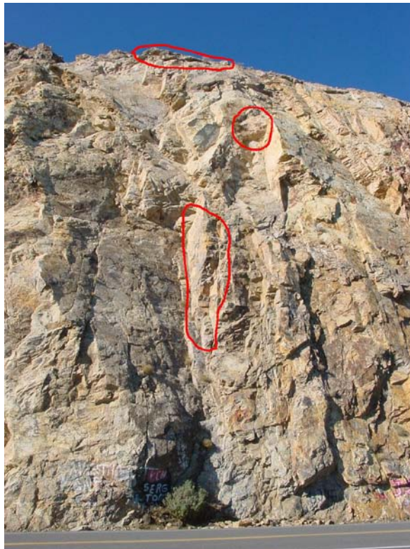
Fig 6. Milepost 63.33 showing fractured rock wedges and soil overhang. Note rock debris in roadside ditch from recent rock fall.
