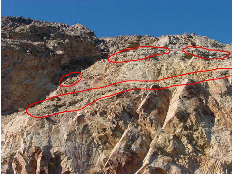
Fig 15. Milepost 63.70 showing perched rocks and soil mass at midslope bench and soil overhangs at crest.
