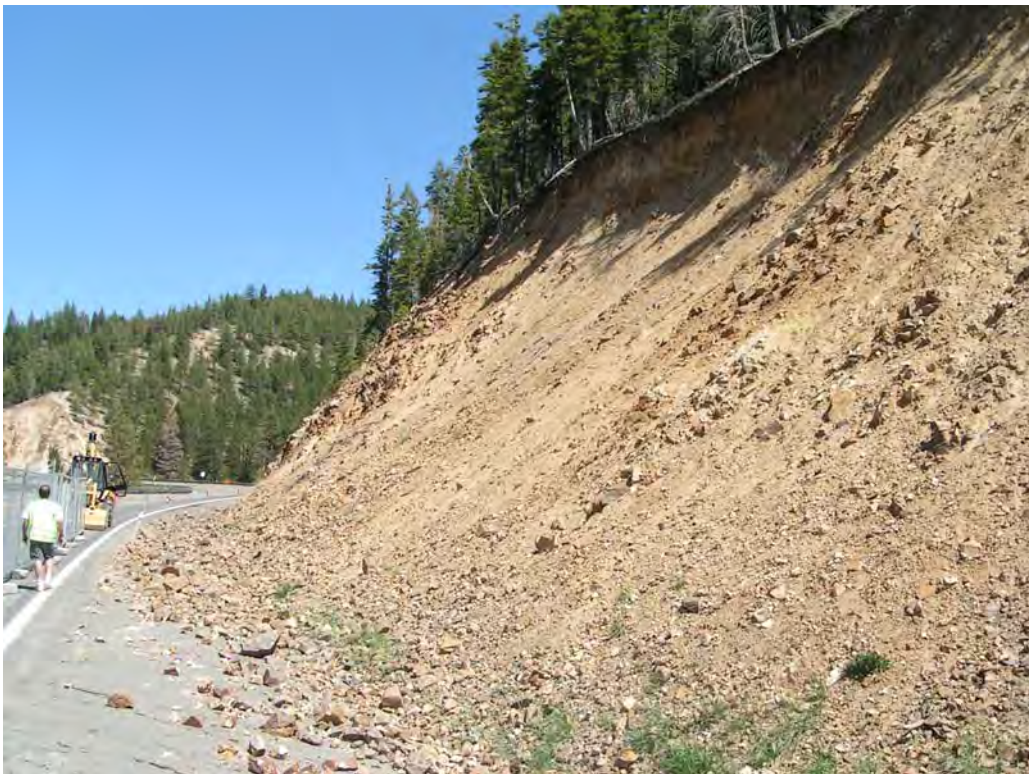
Debris along the toe of Slope 27
