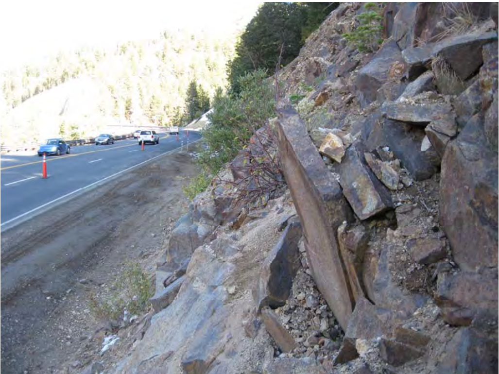
Example of toppling failure in Slope 27
