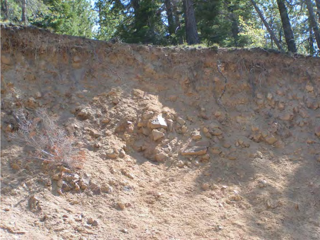
Upper portion of Slope 27 is a mix of soil and rock and undercuts the soil
