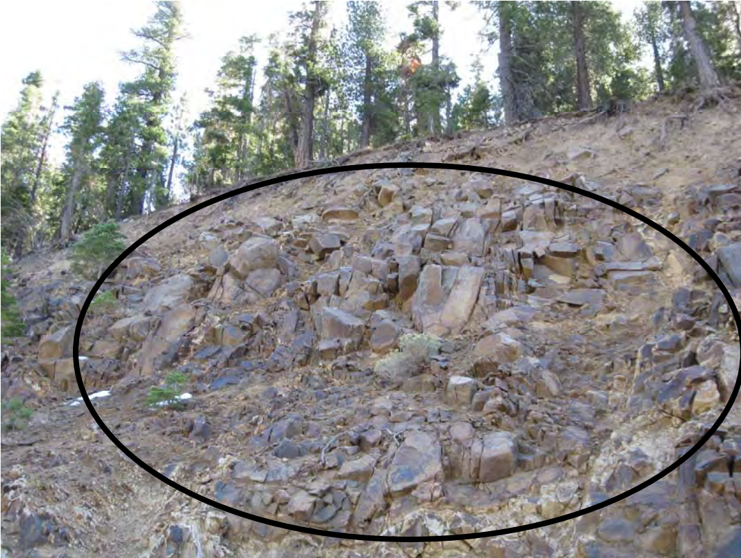
Rock will be required to be scaled from portions of Slope 27
