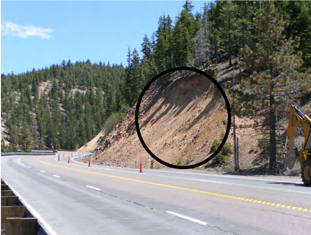
Slope 27 looking east along Hwy 50 – circled area exhibits slide failures
