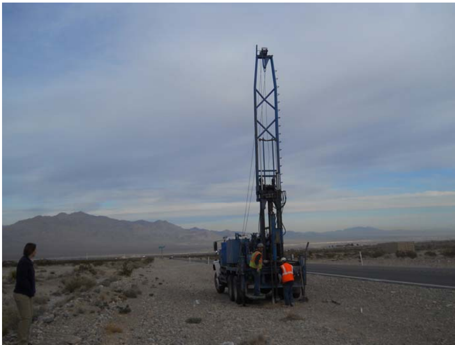
YA-08 – Kyle Canyon Road near Lucky Star Road – Westbound
