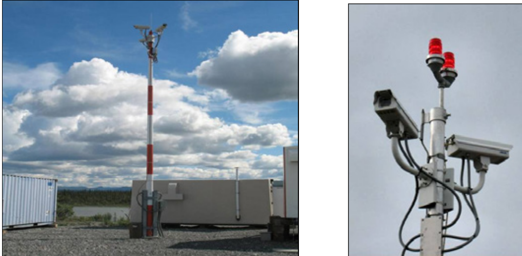
Figure 6-34. Weather Camera (WCAM) pole
