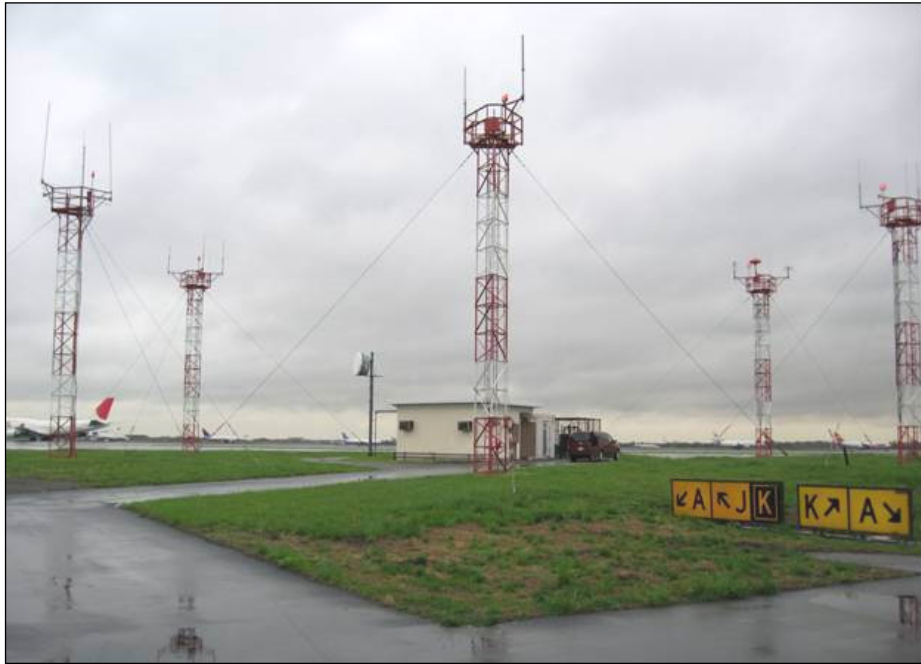
Figure 6-4. Remote Transmitter/Receiver (RTR) communication facility
