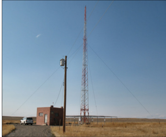
Figure 6-31. Non-Directional Beacon (NDB) facility
