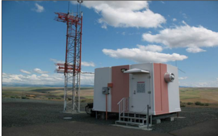
Figure 6-24. GS antenna and equipment shelter
