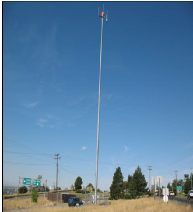
Figure 6-36. Low Level Windshear Alert System (LLWAS) sensor pole
