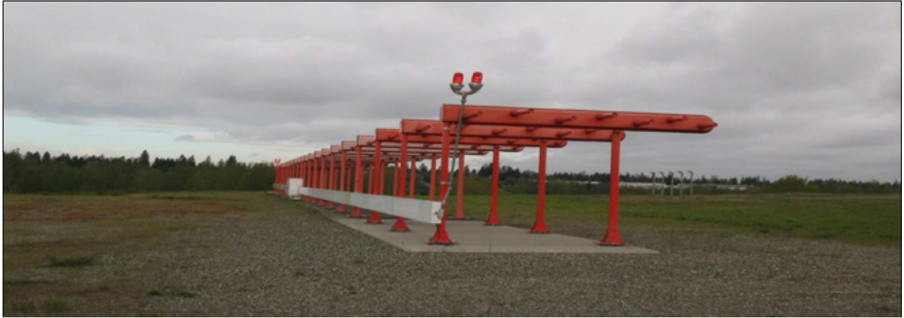
Figure 6-22. LOC 14-antenna array
