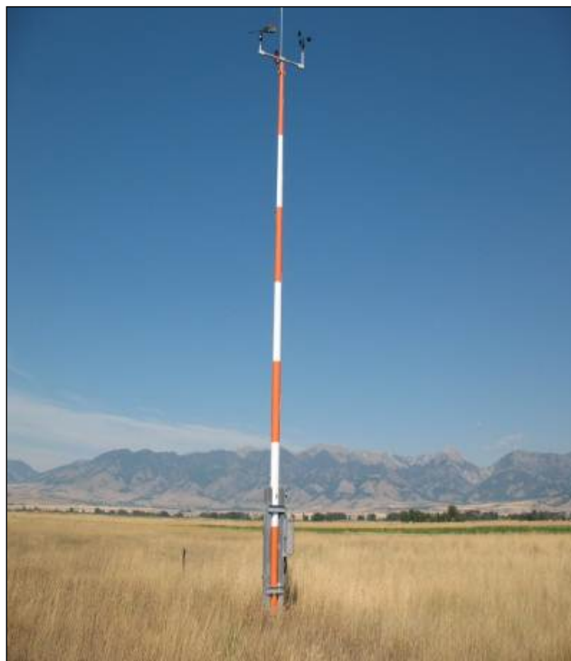
Figure 6-35. Weather equipment sensor pole
