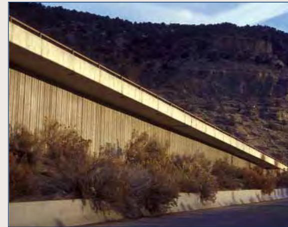
(2) An example of a cantilevered retaining wall with a simple, consistent use of materials. Vertical joints are most compatible with the finish.
