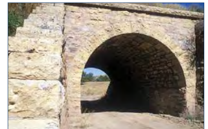
(6) Native materials can be used to create unique pedestrian undercrossings. In this example, the height of the opening allows light into underpass.
