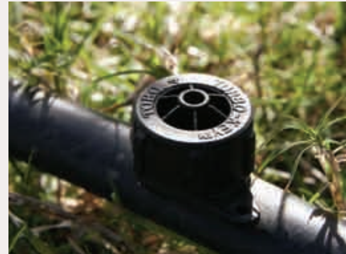
(1) Drip irrigation is required for all enhanced native, regionally adapted, and regional ornamental softscape types even after they have reached maturity.
