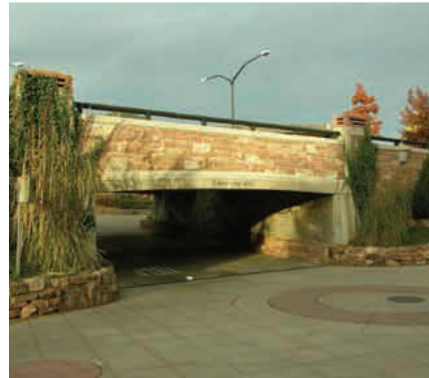
(1) The length of underpasses should be minimized where possible in order to allow natural lighting.
