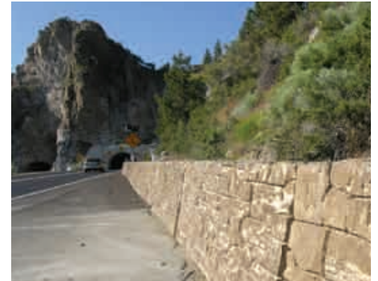
(2) Colors and simple patterning of walls and barrier rails should be the standard in areas of national significance.
