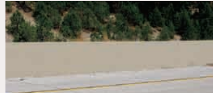
(1) Stained concrete barriers should use colors from the design segment’s color palette.
