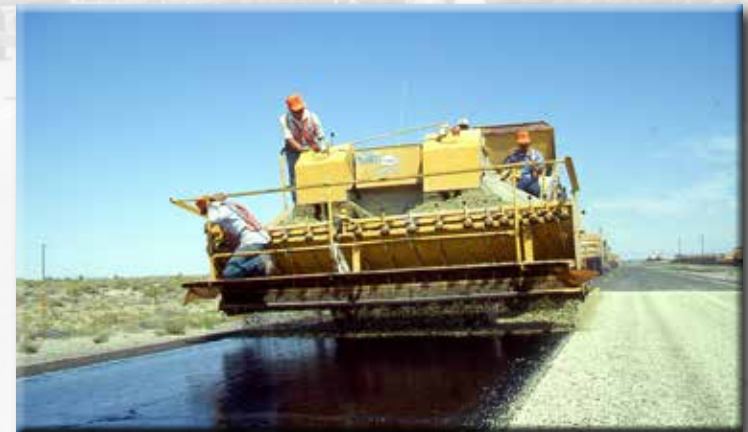
Paving continued in the 1980s on U.S. Highway 50, also known as the "Loneliest Road in America"
