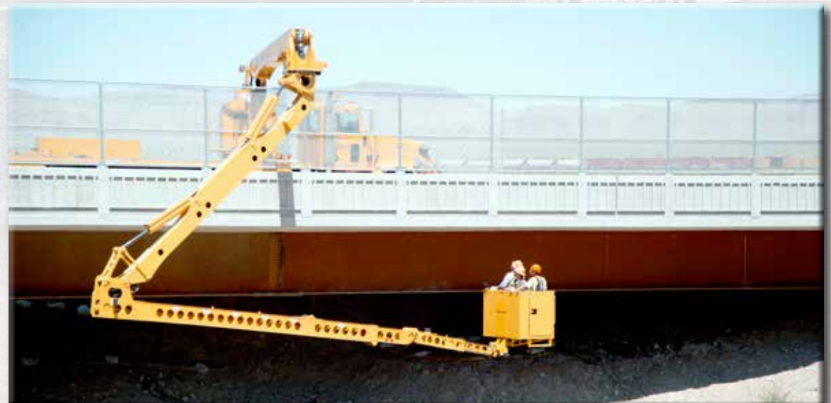
The department inspects its bridges every two years. A Dunphy Bridge inspection is shown here in 2015
