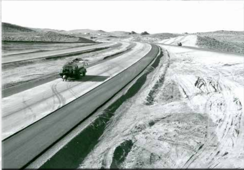
U.S. Highway 50 was named "America's Lonliest Road" by Life Magazine in 1986. Pictured is the construction of the highway
