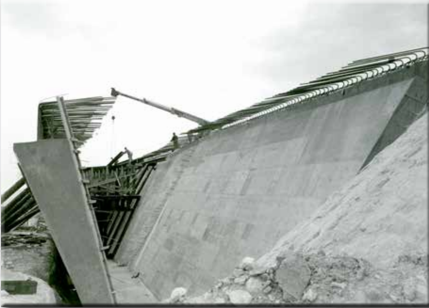
The Monrow Construction Company works on the Bonanza Road Expressway in Las Vegas
