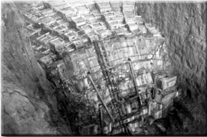
Dam forms are squeezed into Black Canyon to begin construction of the Boulder Dam
