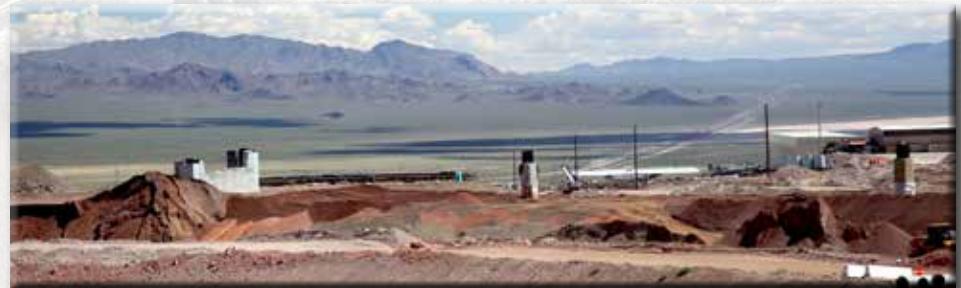
In 2015, NDOT broke ground on Interstate 11, a route that will connect two cities – Phoenix and Las Vegas. The interstate will bypass Boulder City, alleviating traffic jams through downtown
