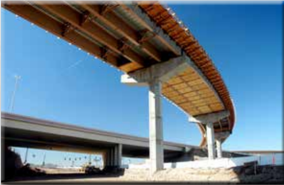
The Henderson "Spaghetti Bowl" opened in 2006, linking Clark County 215 with U.S. Highway 95
