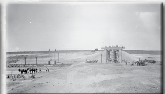
Early roadway construction included grading through wide swaths of barren desert land
