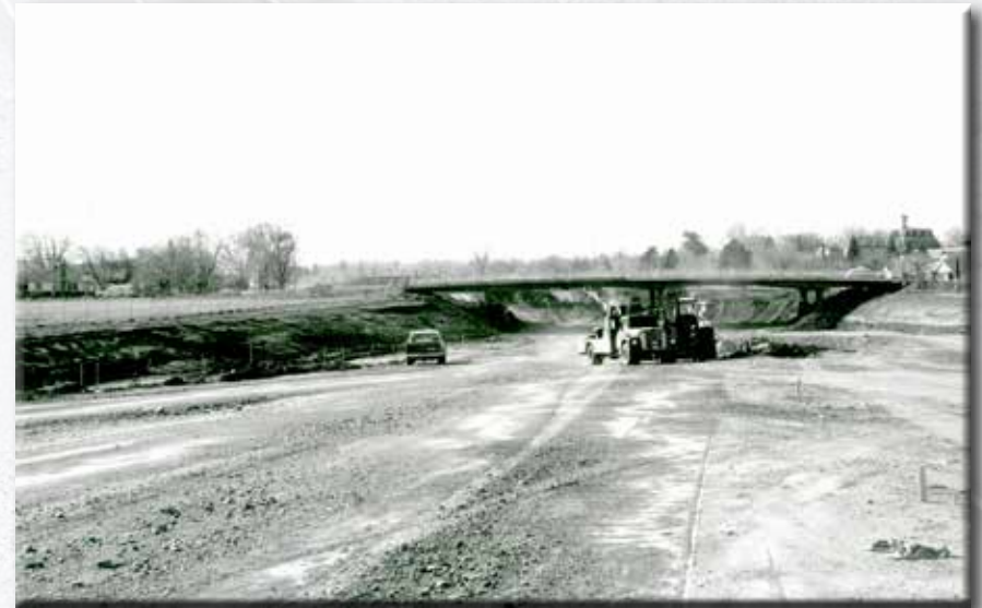
Construction takes place on Interstate 80 in Reno, an important route that stretches from the ports of Oakland, California
