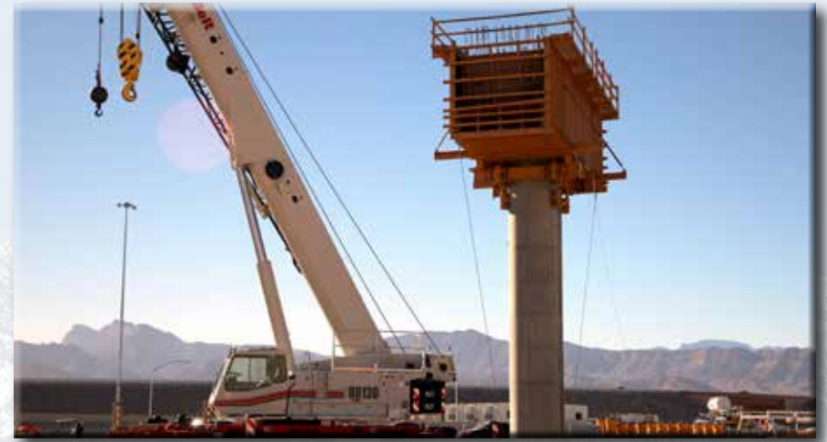
The Centennial Bowl, shown here under construction here in 2015, will accommodate motorists in the fast-growing northwest region of the Las Vegas Valley
