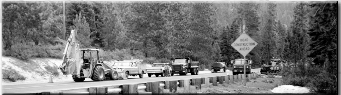
Crews work on State Route 28, the link between U.S. Highway 50 and the California state line
