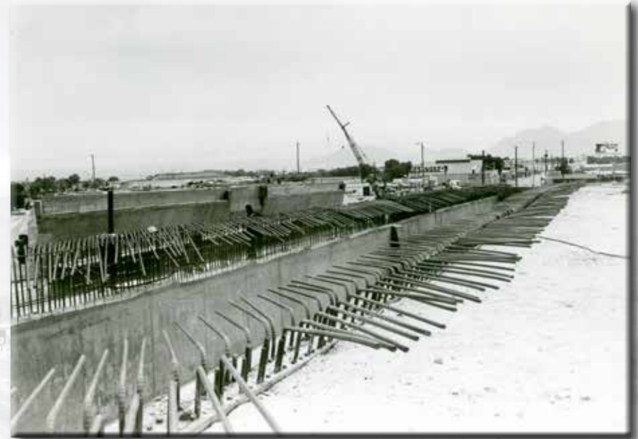
The Monrow Construction Company works on the Bonanza Road Expressway in Las Vegas
