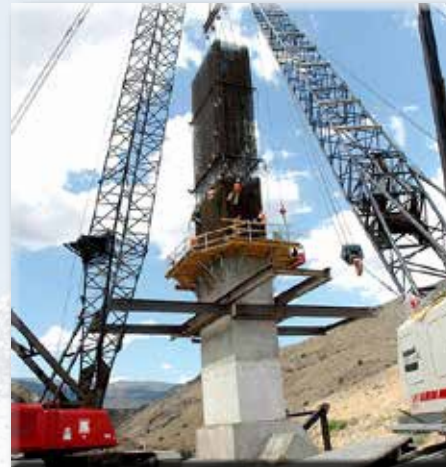
The Galena Creek Bridge in northern Nevada was one of the department's largest undertakings
