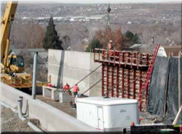
After traffic volumes climbed to 233,000 a day, the department embarked on a $53 million makeover of the Reno Spaghetti Bowl in 2002
