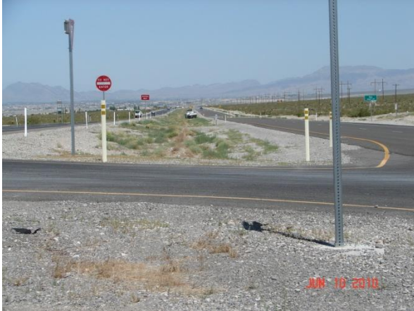
At station "P" 318+79 at CPB12 looking west towards the end of project.
