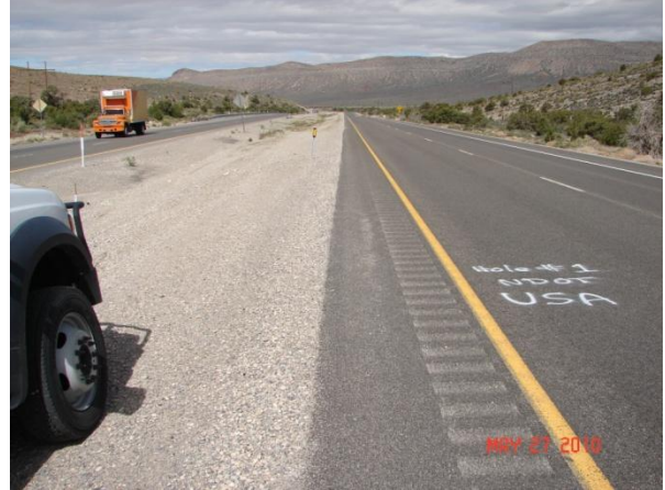
Beginning of project at station "X2" 1140+67 at CBP1 looking west along project alignment.
