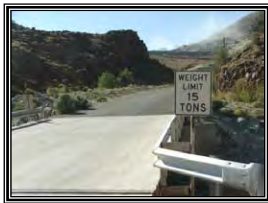
Example of Structurally Deficient Bridge
