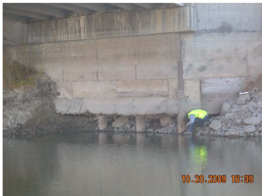
Eden Valley Bridge B-1658 -Scour
