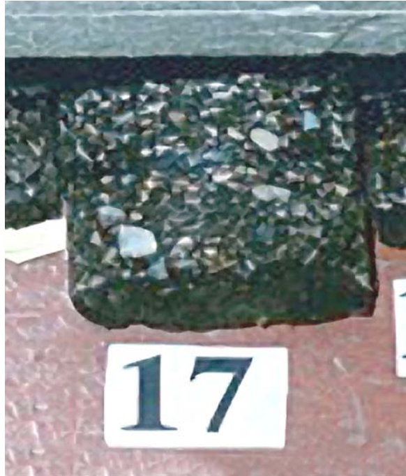
Before Construction: Light Stripping Pavement Condition: High Severity Transverse Cracking
