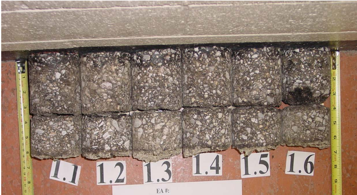
(a) 2 Years after Construction: Delaminated at 3.6 in. with Light to Medium Stripping Pavement Condition: Good Condition
