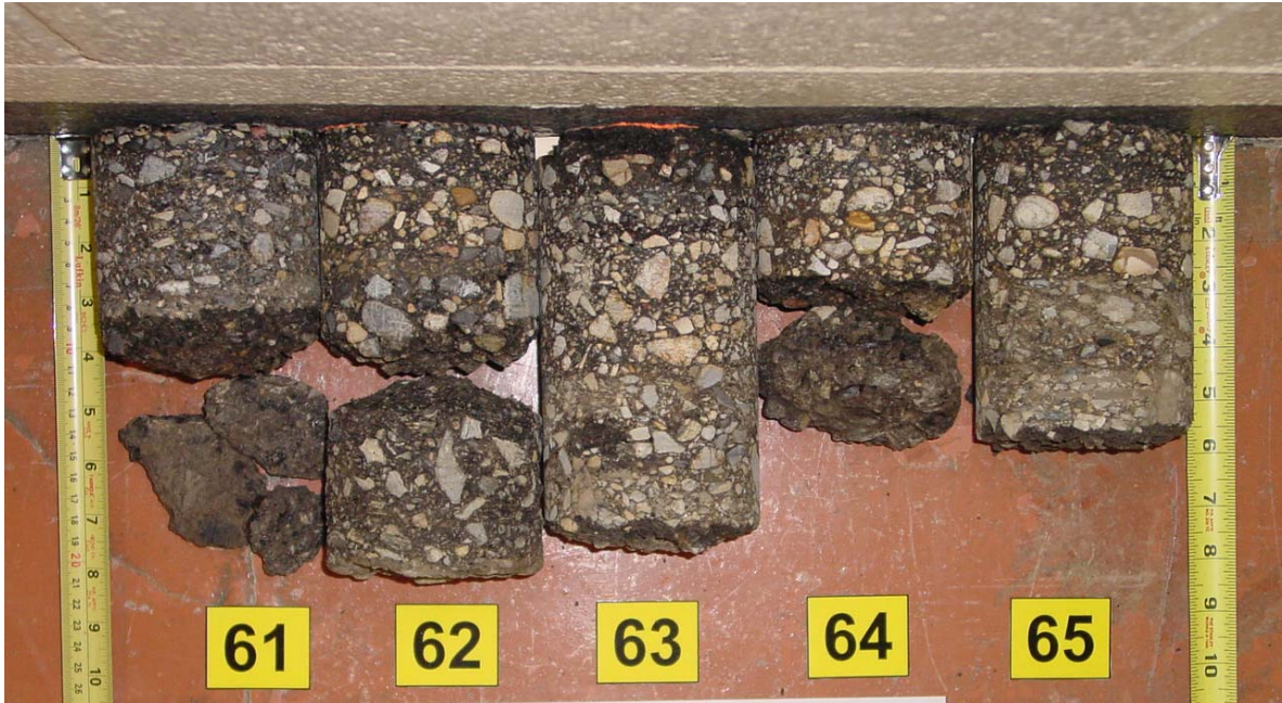
Before Construction: Light to Heavy Stripping and Fell Apart Pavement Condition: Transverse and Nonwheel Path Cracking
