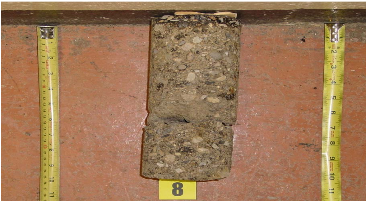
3 Years after Construction: Broke from 6.0 in. to 7.3 in. Pavement Condition: Low Severity Transverse Cracking
