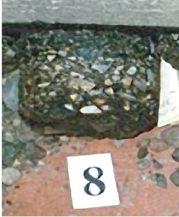
Before Construction: Medium Stripping Pavement Condition: High Severity Transverse Cracking
