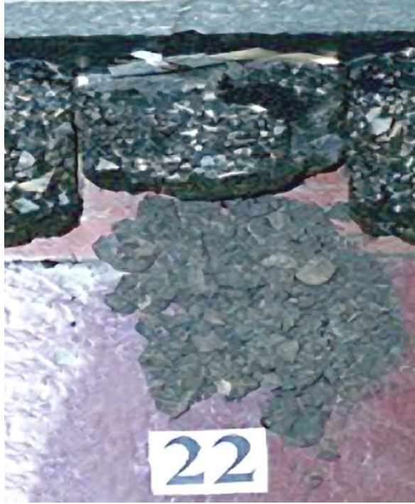
Before Construction: Heavy Stripping and Fell Apart Pavement Condition: High Severity Transverse Cracking
