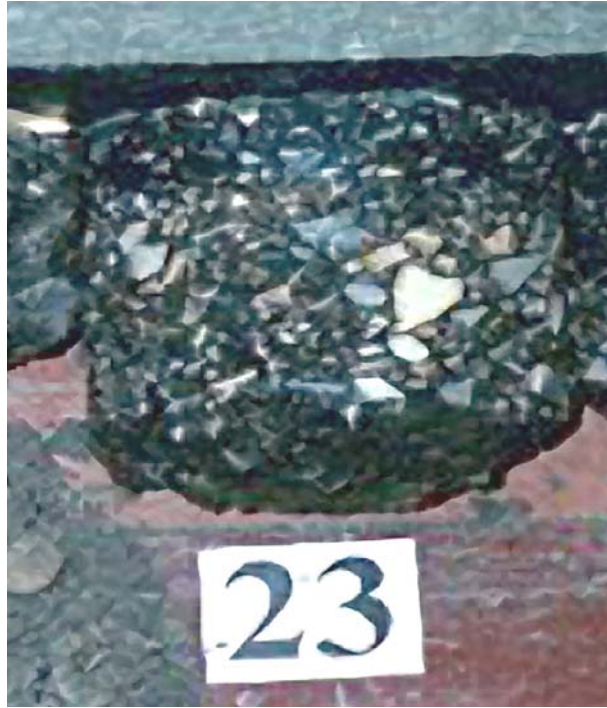
Before Construction: Heavy Stripping Pavement Condition: High Severity Transverse Cracking
