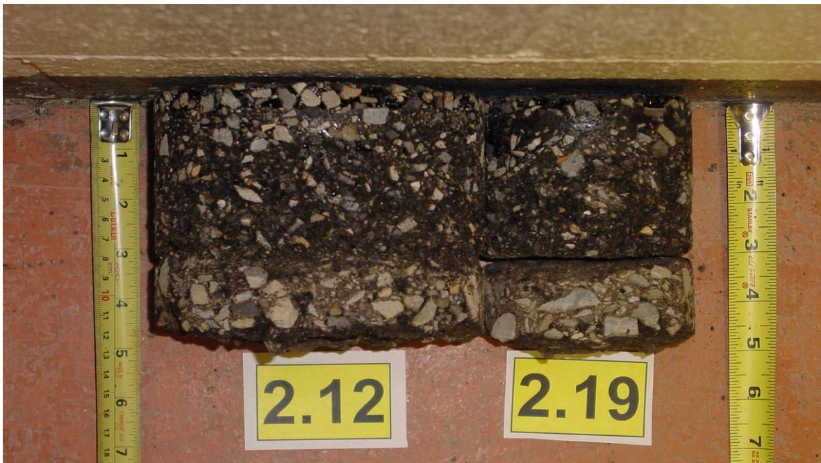
1 Year after Construction: Light to Medium Stripping and Delaminated at 3.0 in. Pavement Condition: Good Condition
