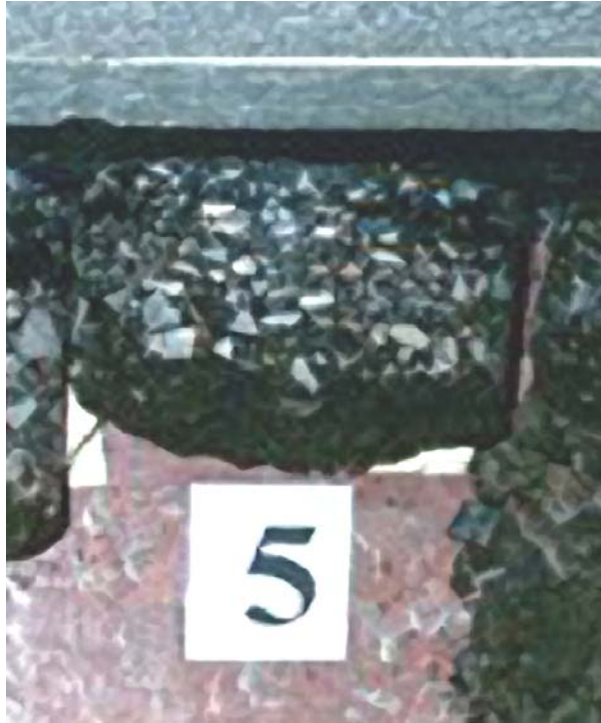
Before Construction: Stripped and Fell Apart Pavement Condition: Transverse and Fatigue Cracking
