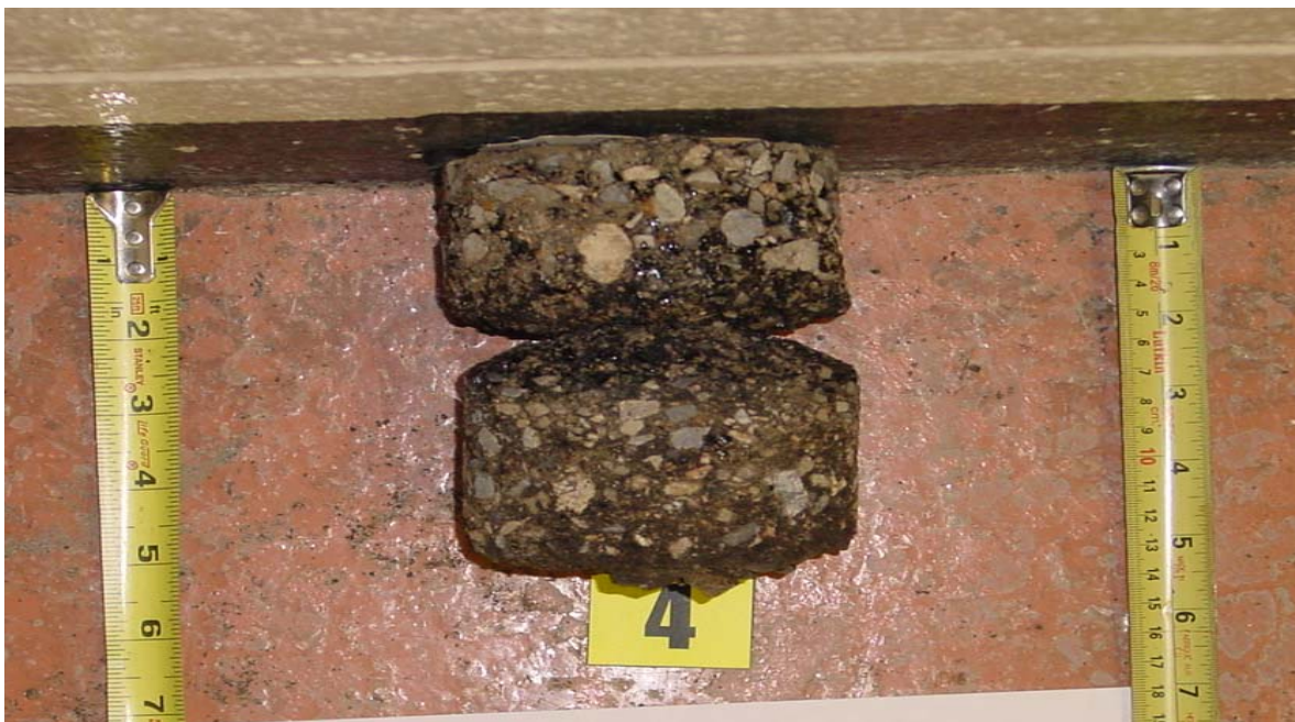
3 Years after Construction: Delaminated at 2.3 in. with Medium to Heavy Stripping Pavement Condition: Good Condition
