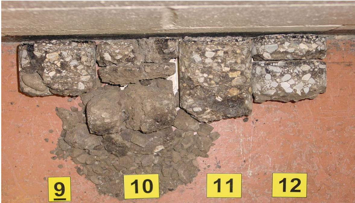
Before Construction: Light to Heavy Stripping, Delaminated, and Fell Apart Pavement Condition: Transverse and Block Cracking
