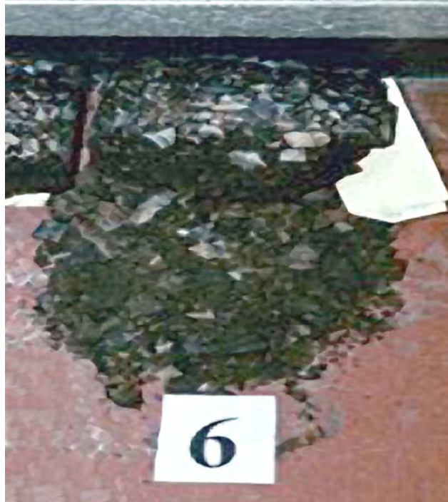
Before Construction: Heavy Stripping and Fell Apart Pavement Condition: Fatigue Cracking
