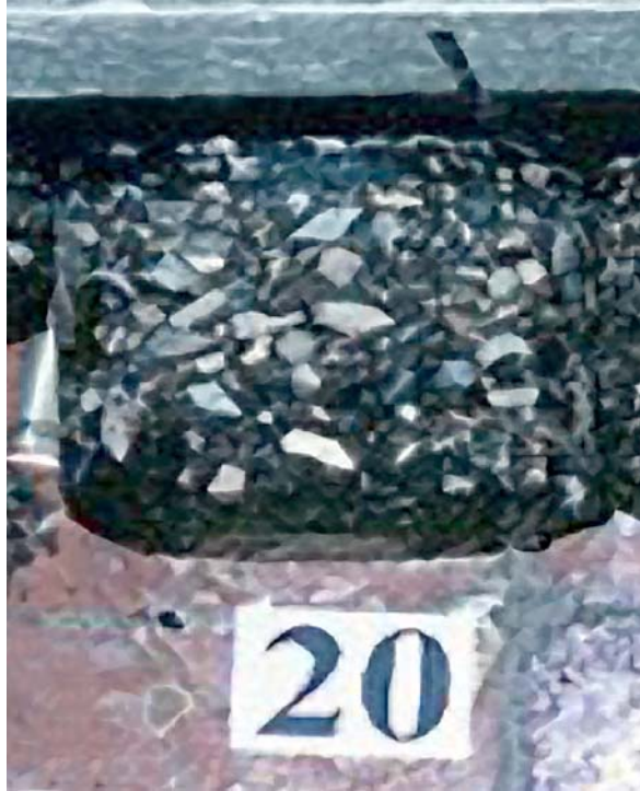
Before Construction: Medium Stripping Pavement Condition: Fatigue Cracking
