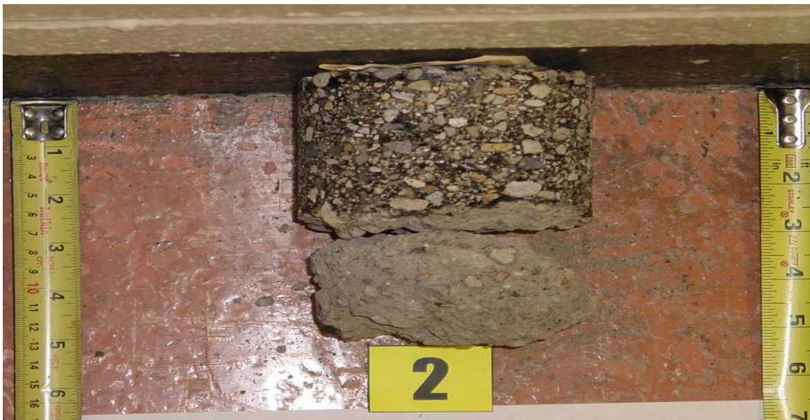
3 Years after Construction: Broke at 2.25 in. Pavement Condition: Low Severity Transverse Cracking
