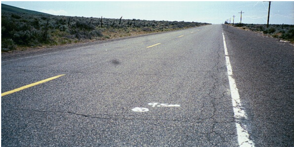
FIGURE 1.2a Common low-volume road distresses.
