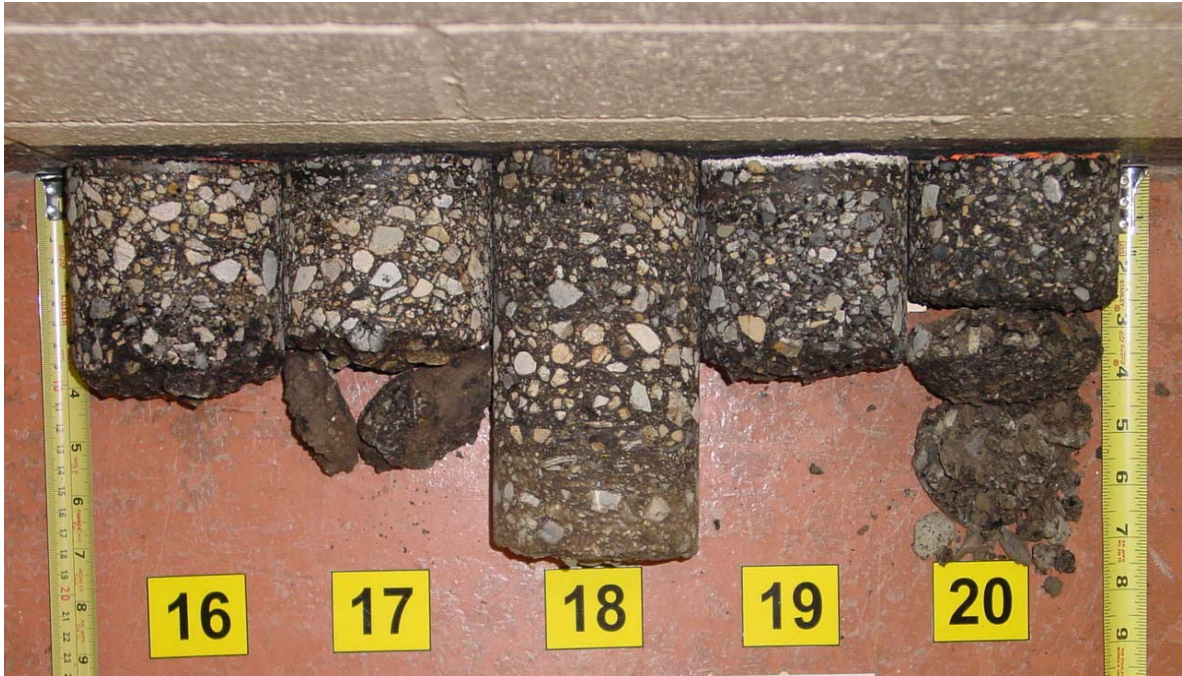
Before Construction: Light to Heavy Stripping, Delaminated, and Fell Apart Pavement Condition: Transverse and Nonwheel Path Cracking
