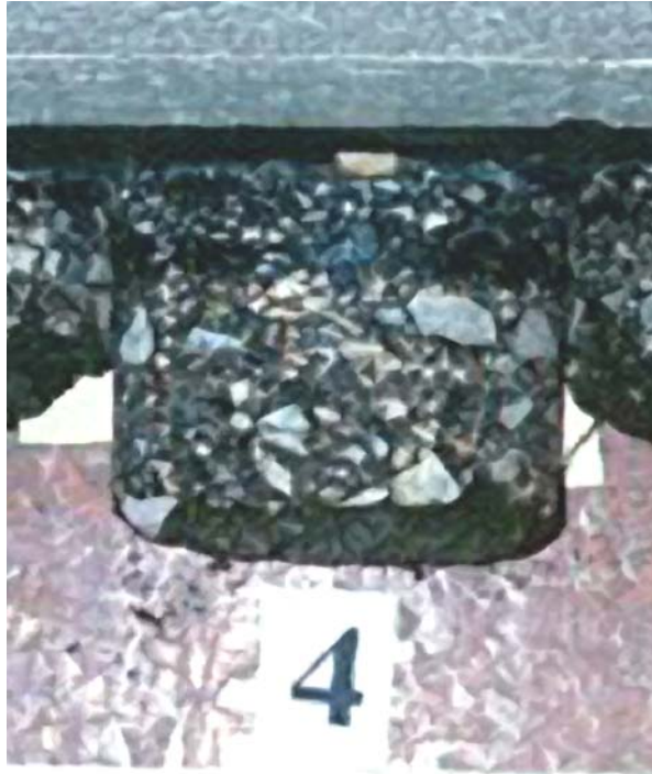
Before Construction: Medium Stripping Pavement Condition: High Severity Transverse Cracking
