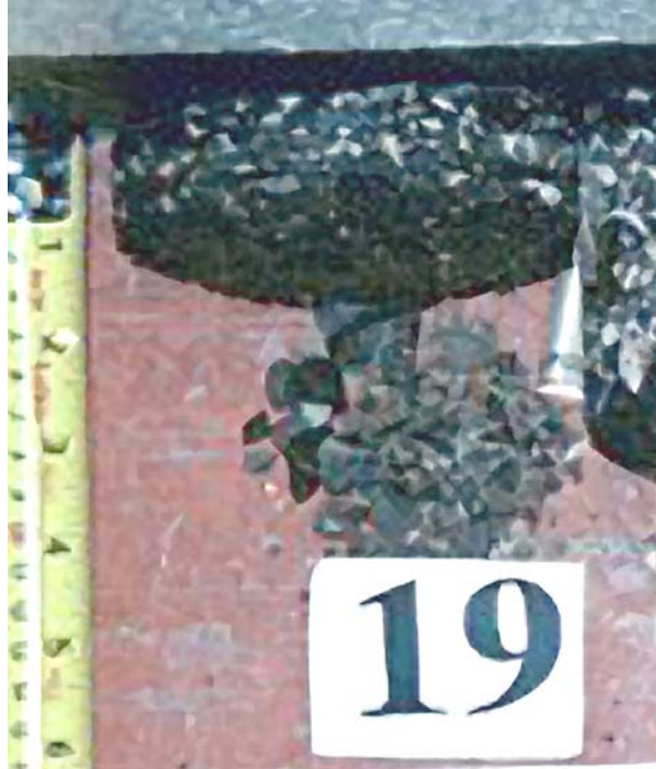
Before Construction: Stripped and Fell Apart Pavement Condition: Transverse and Fatigue Cracking
