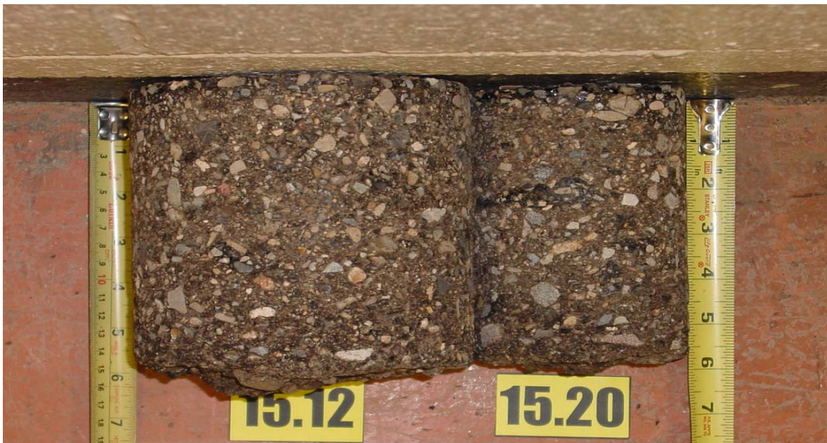
3 Years after Construction: Light to Medium Stripping Pavement Condition: Low Severity Transverse Cracking
