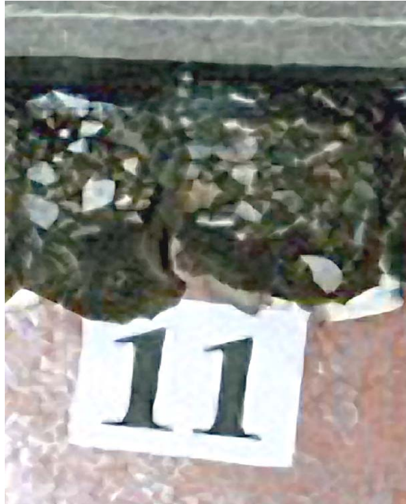
Before Construction: Heavy Stripping and Fell Apart Pavement Condition: Transverse and Fatigue Cracking
