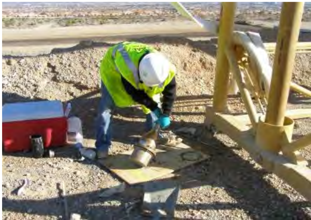
Figure 6.20: Volumetric air content test for post-pumped SCC
