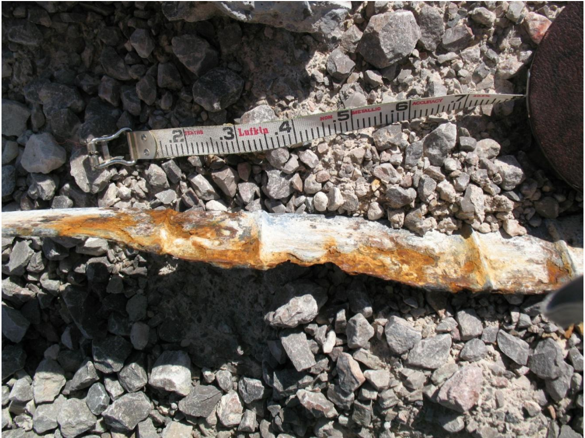
Figure 47. Cheyenne MSE Wall Corrosion Investigation - Highly Corroded Reinforcing Strip
