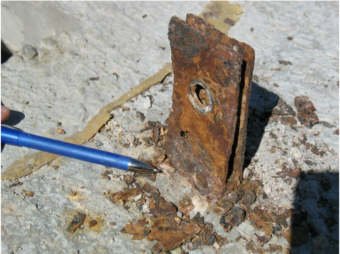
Figure 50. Cheyenne MSE Wall Corrosion Investigation - Corroded Steel Facing Connection
