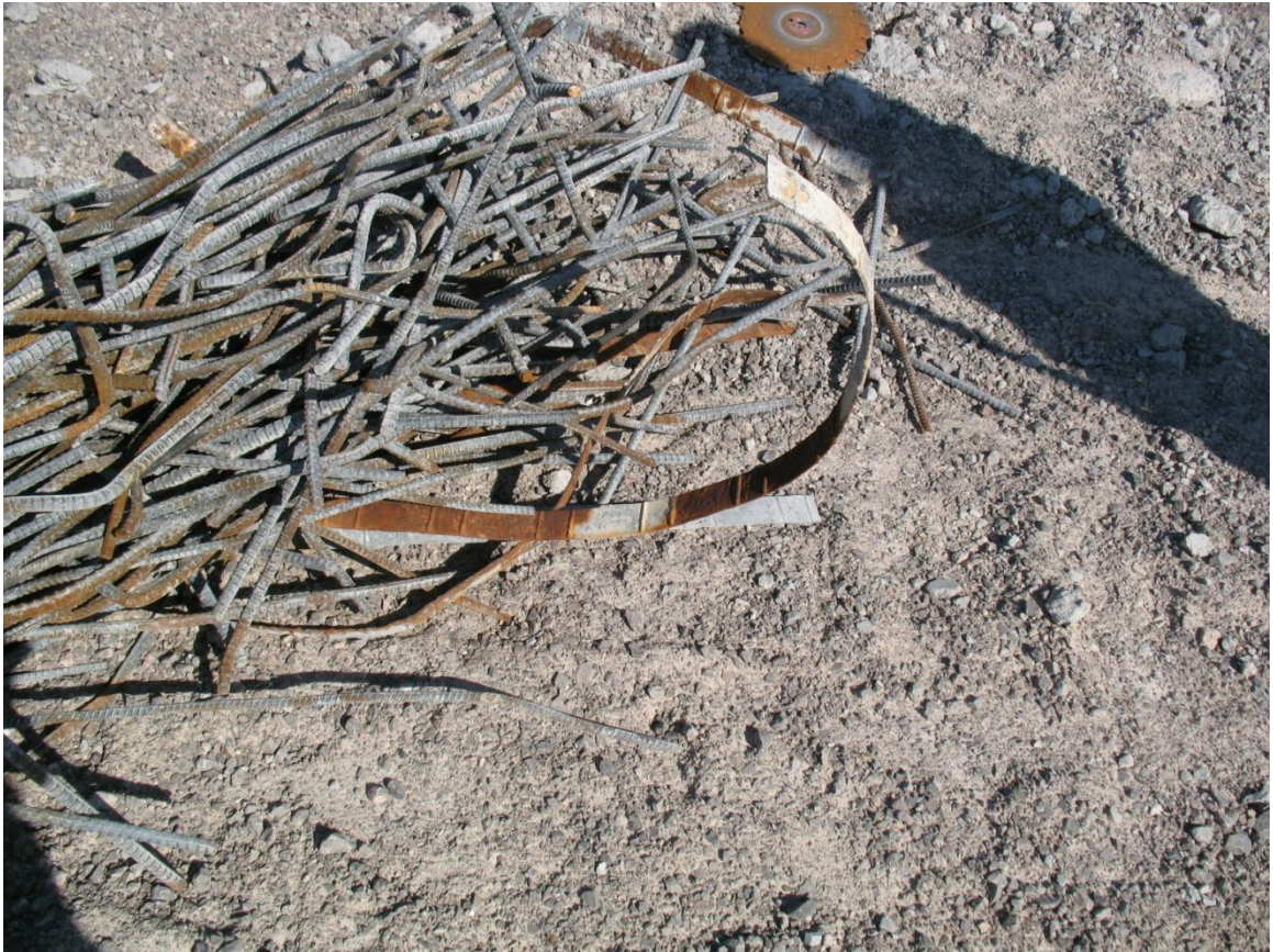
Figure 48. Cheyenne MSE Wall Corrosion Investigation - Reinforcing Strips in Pile of Debris
