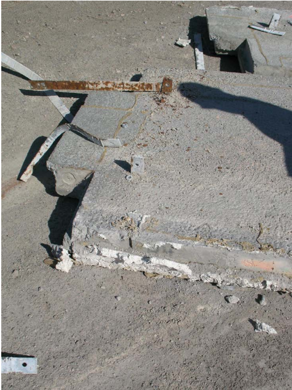
Figure 49. Cheyenne MSE Wall Corrosion Investigation - Styrofoam at Top End of Panel
