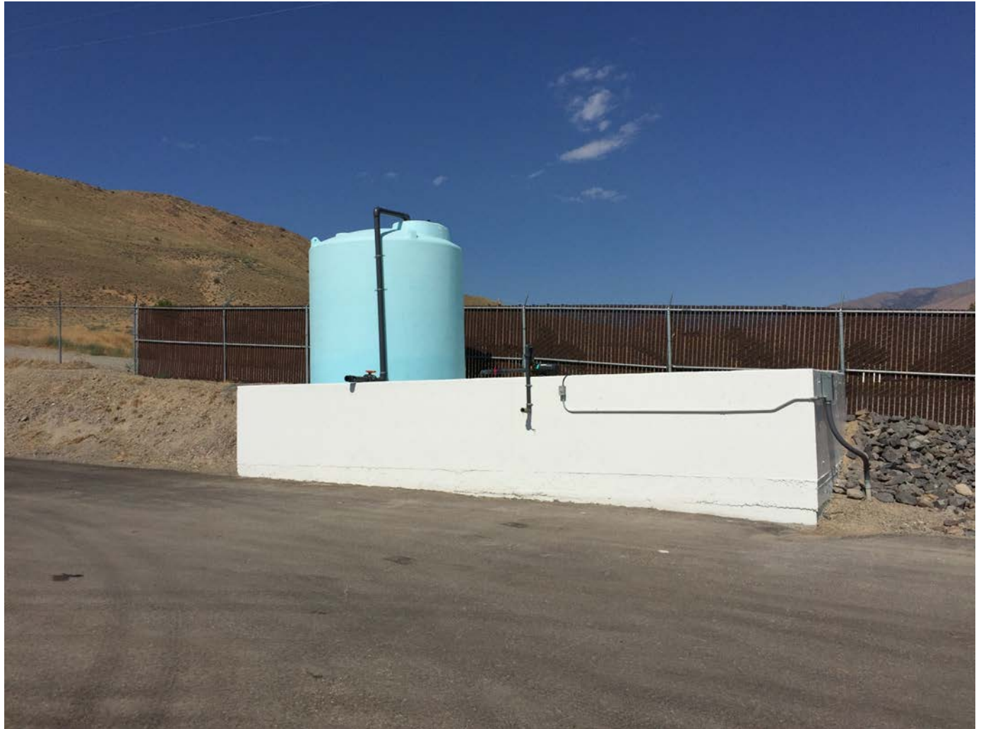
Brine tank secondary containment structure (Wellington Station)
