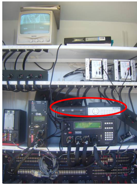
Figure 3-3 DVR Setup in a Traffic Signal Cabinet
