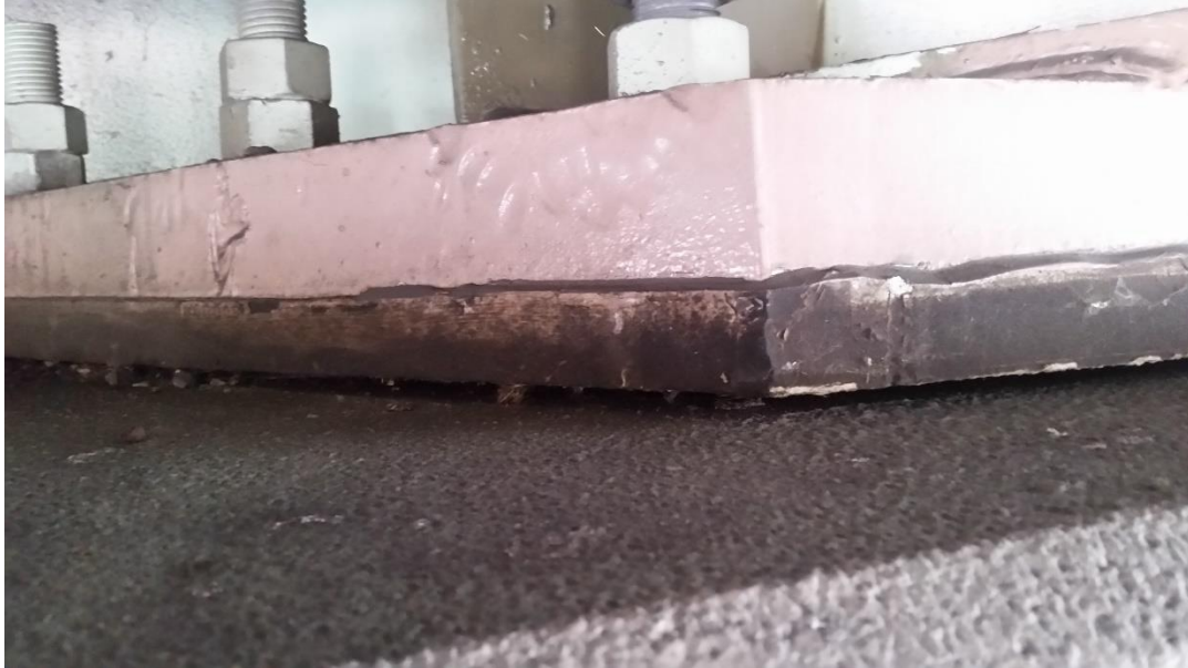
Figure 6-18: Bearing 7 of Abutment 2 partial uplift from substructure
