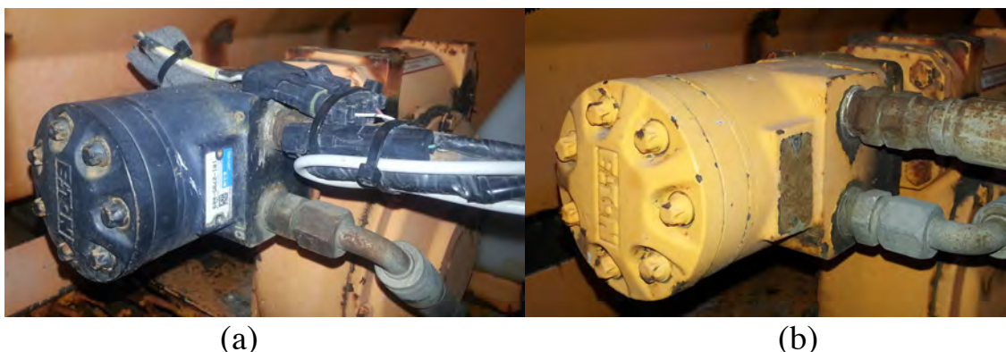
Figure 3.4: The Eaton 10903 W/S hydraulic motor installed on an NDOT dump truck spreader system (a). This motor included a three-wire harness that allow for the observation of the motor's speed, while standard hydraulic motors (b) did not contain such a wiring harness.
