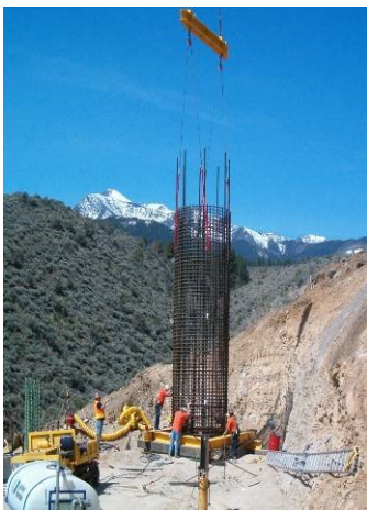
Figure 47: Construction of a drilled shaft foundation with installation of a reinforcing steel cage
