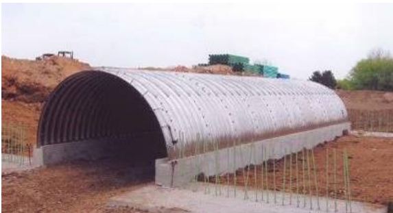
Figure 51: Metal arch pipe
