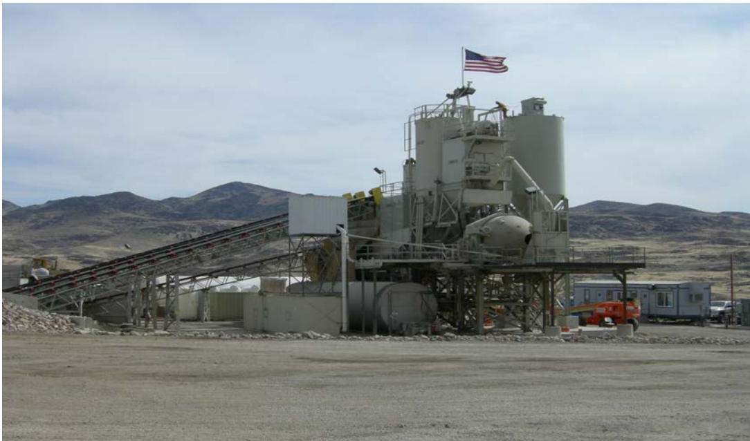
Figure 26: Central-mix type concrete mixing plant
