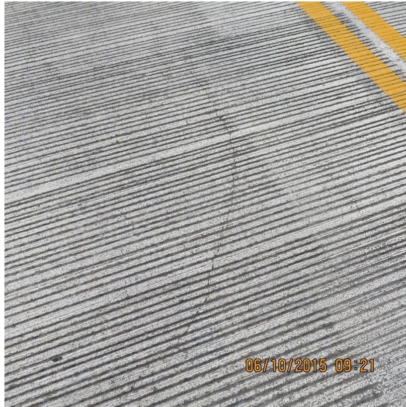
Figure 3-8. Bridge deck of bridge H-2285 with some visible cracking.
