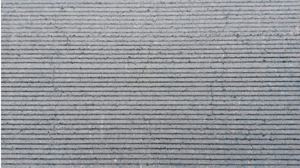
Figure 3-12. Close-up of cracking on eastern deck showing fine cracks.
