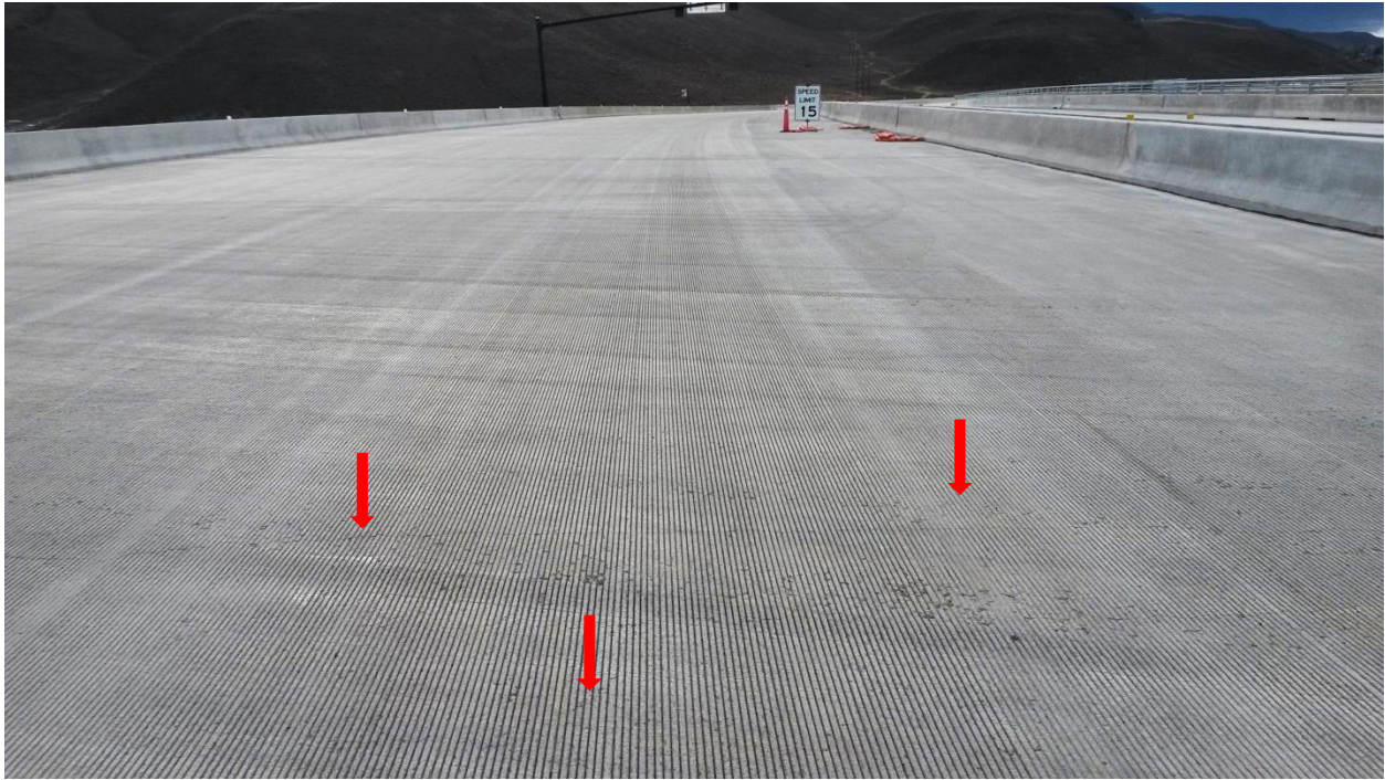
Figure 3-10. View looking south on eastern deck of SE Connector with visible cracking that is difficult to see.
