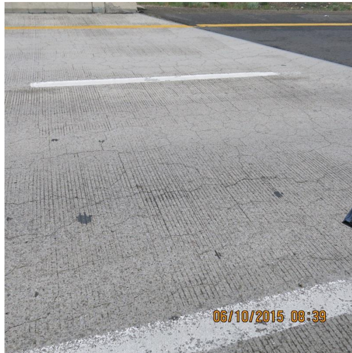
Figure 3-2. Bridge H-2298 bridge deck. Note high density random cracking throughout.
