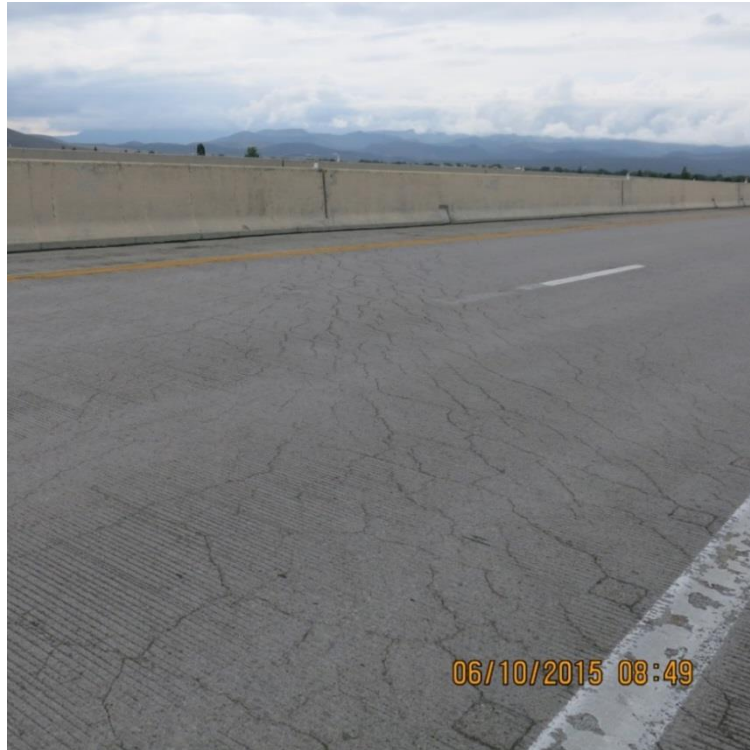
Figure 3-3. Bridge I-2296 bridge deck. Note the high density random cracking throughout, with some cracking oriented above underlying skewed pier.
