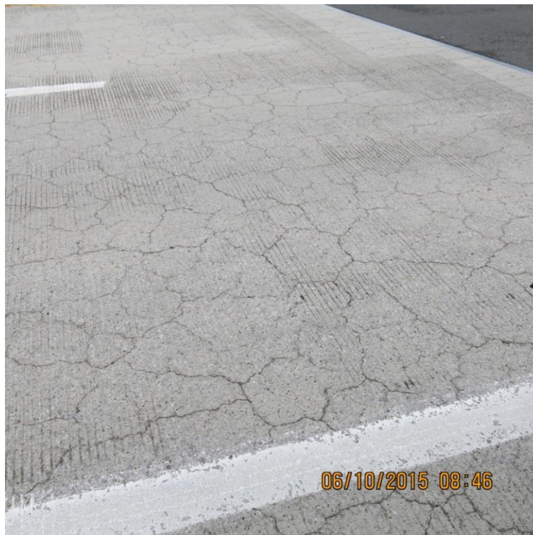
Figure 3-4. Bridge H-2297 bridge deck. Note high density random cracking throughout.
