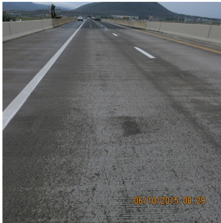
Figure 3-5. Bridge I-2293 bridge deck with visible cracking throughout.
